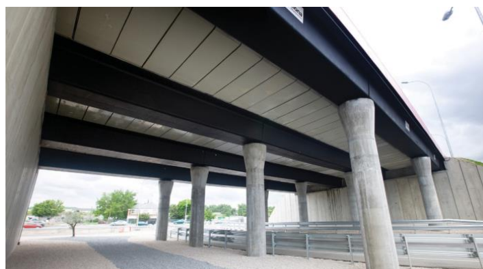
Figure 17. M111 road bridges, Madrid, Spain, consisting of moulded FRP primary beams and concrete deck, were built in 2007 [65,68].
