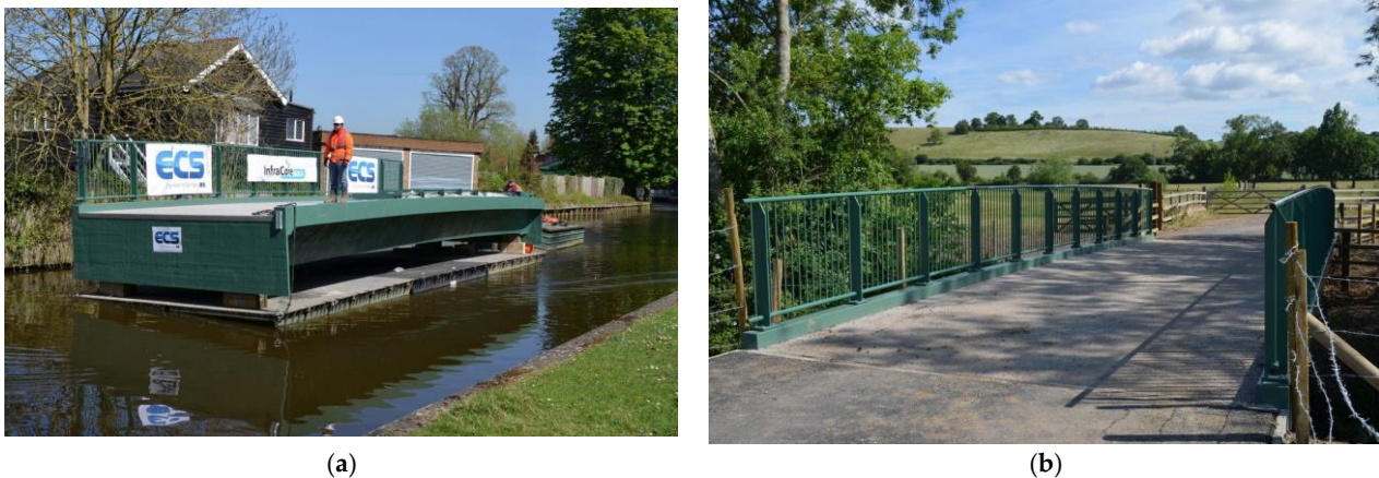
Figure 21. Mapledurham Footbridge, Mapledurham, Oxfordshire, UK, built in 2015 [8]: (a) FRP bridge deck delivered to site by floating on a barge along River Thames; (b) Mapledurham FRP bridge installed with no physical joints.
