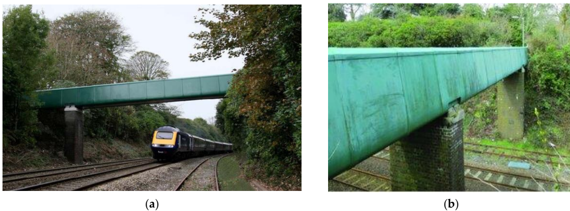
Figure 9. St Austell Railway Bridge, Cornwall, UK, built in 2007 [56]: (a) Front view of the bridge; (b) Side view of the bridge.
