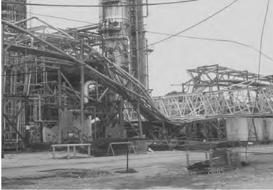
Figure 1.1: Damaged Pipe Rack - Hurricane Rita (Photo Credit: Louisiana Chemical Association)
