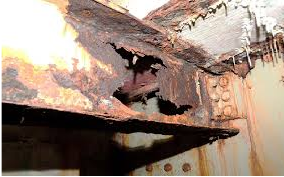
Figure 5.1: Corrosion issue of a steel structural member
