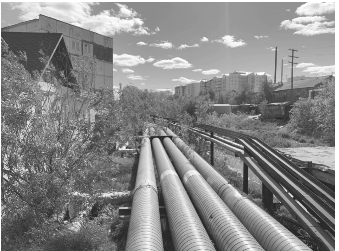
Fig.1-5 - The Centralised Heating Pipe System along the Canal behind Lermontova Street, Yakutsk
