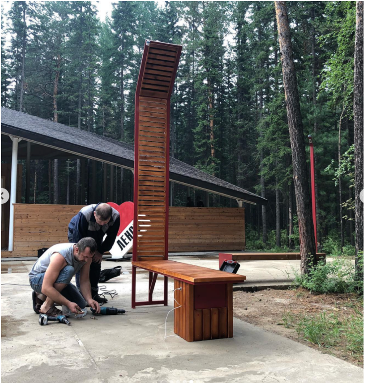
Fig.6-3 - Oyuur Park –Men Building an Experimental Bench Initiated by Local Participants After the Park Project was Built
