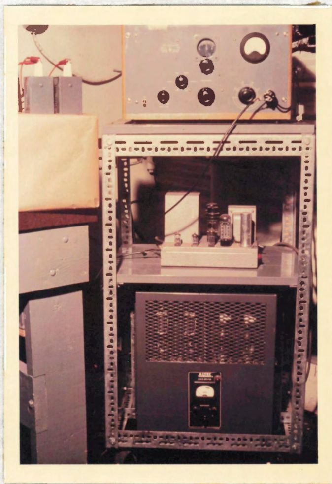
Figure 6. The voltage and frequency generating equipment.
