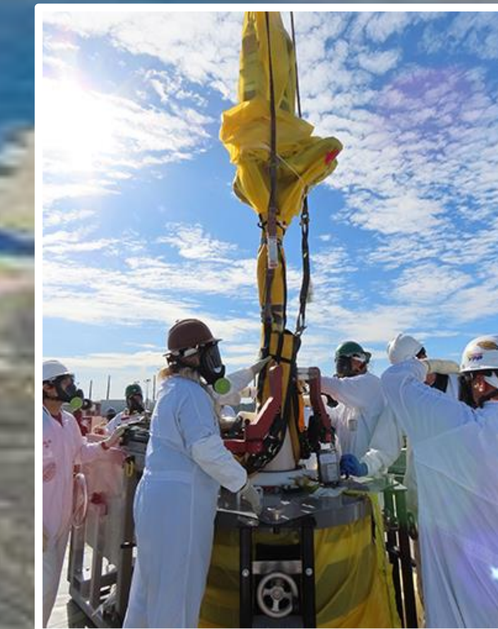
Figure 5: Cleanup workers replacing a pump where nuclear waste is placed before treatment and vitrification (Hanford Site)
