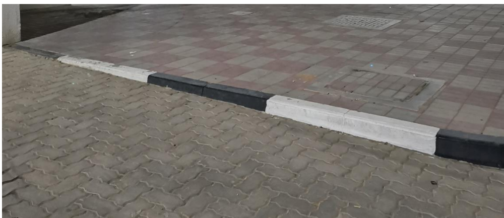
Figure 18: Slope in the Sidewalk at the Entrance of Every Villa
