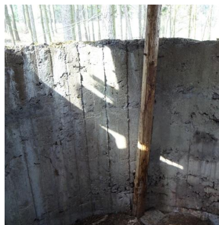
Fig. 6 – Preserved original shaft from 1938 in the western wing of the pillbox T-S 20.
