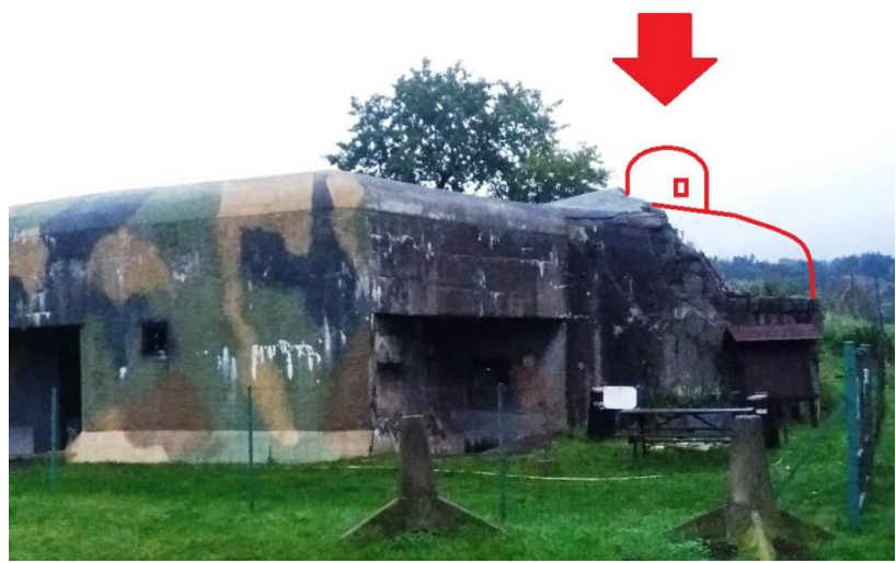
Fig. 2 – Damage of the pillbox by the explosive used for cloche removal during occupation by Nazi Germany in 1939-1945 (pillbox N-S 84 „Voda“ in Náchod, Czech Republic)
