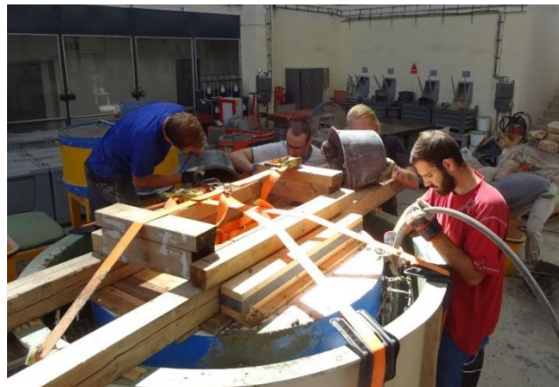
Fig. 10 – Concreting of the cloche after turning the completed mold parts (Laboratory of the Faculty of Civil Engineering, CTU)
