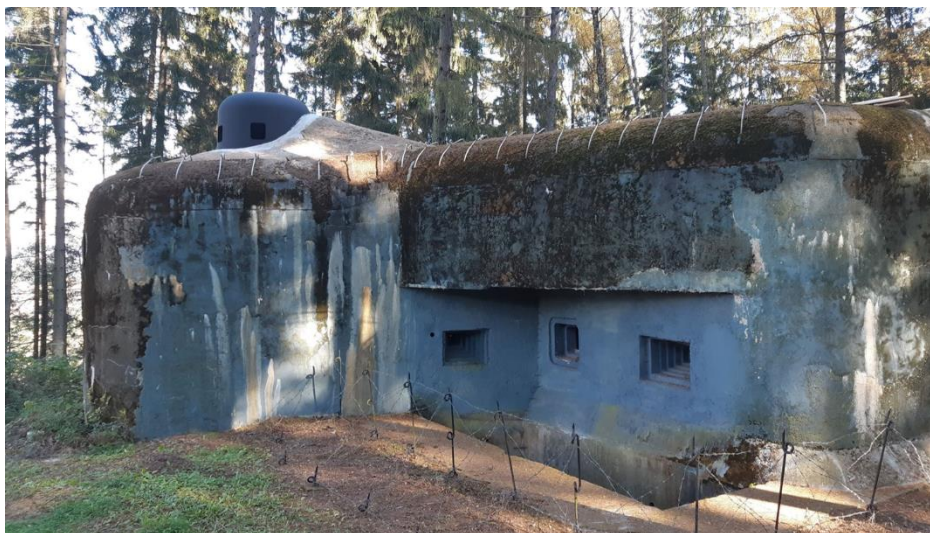
Fig. 19 – Current state of the pillbox T-S 20 (April 2020). Replica of the cloche was painted by the colour imitating metal, reconstruction of the surface plasters has not been made yet (due to COVID 19 pandemic)
