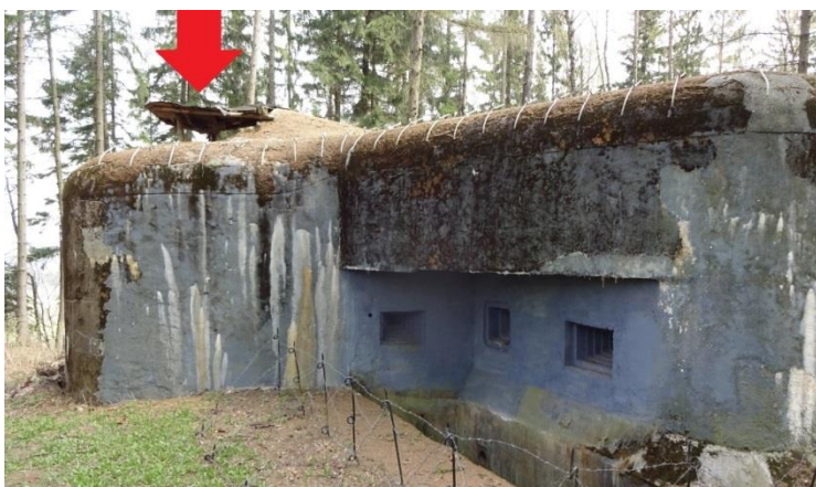
Fig. 5 – Western wing of the pillbox T-S 20. Part for placing the cloche AJ-S-D replica is marked (shaft is covered by wooden construction, which will be removed).
