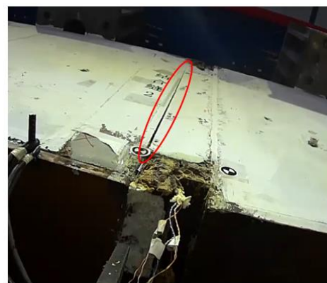
Fig.3-4 Failure state of No.2 seam section
