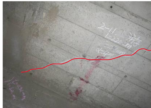
(b) Inclined cracks of the web near the top of No. 11 pier ( L=2.2m \delta=0.18mm \alpha=45^\circ )
