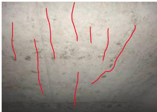
(i) Longitudinal cracks in the roof near of No.10 pier ( L=2.5m \delta=0.2mm \alpha=15^\circ )
