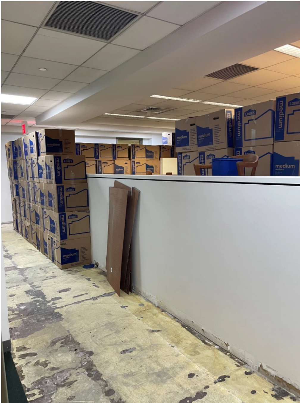
The view from the conference room/temporary office. Boxes contain books temporarily relocated during construction. The carpeting had to be removed due to water damage and is awaiting new carpet installation.
