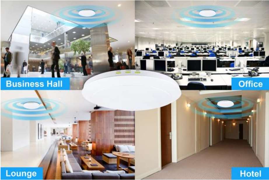
Figure 4.7 Illustration of Wi-Fi access point installed on roof in several areas
