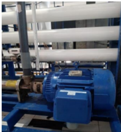
Gambar 10. High Pressure Pump (HPP). Figure 10. High Pressure Pump
