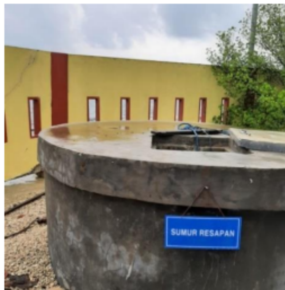
Gambar 3. Sumur resapan untuk proses Intake Figure 3. Infiltration wells for the Intake process
