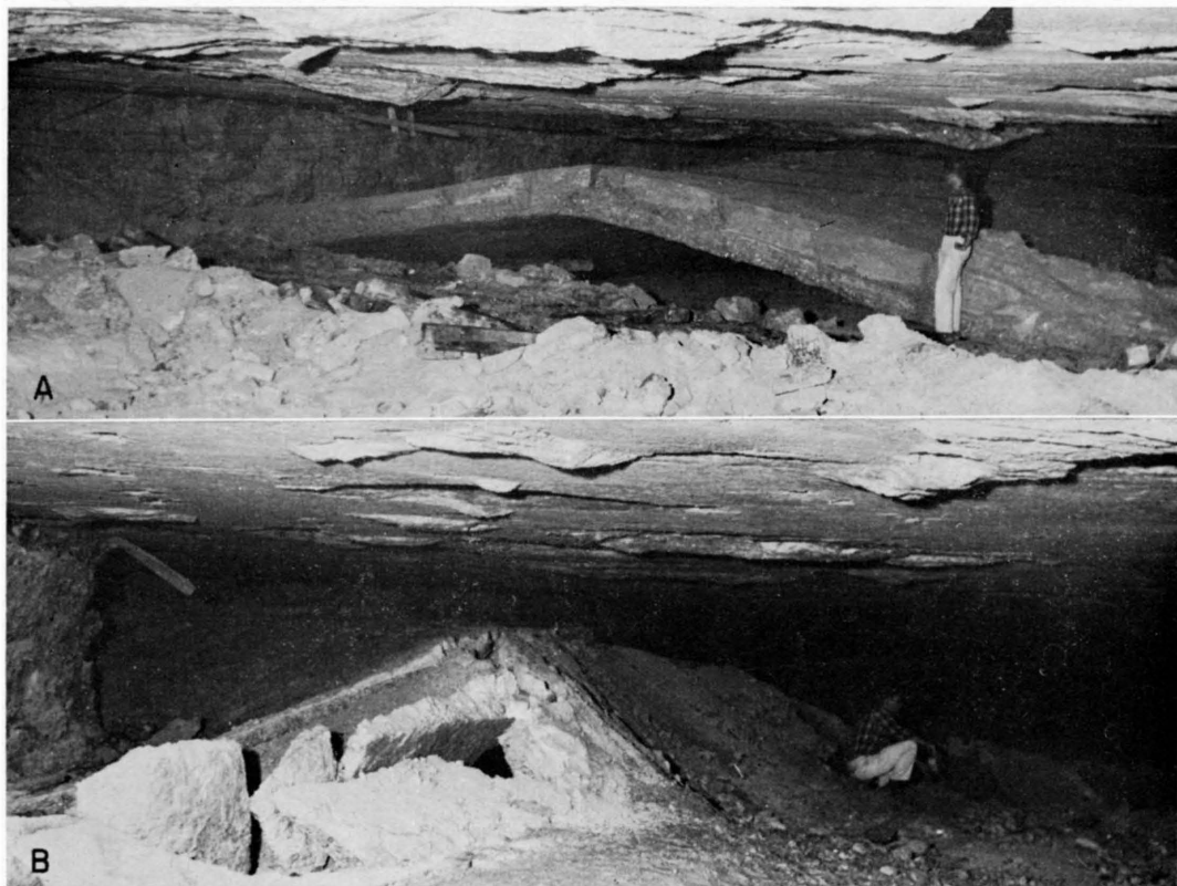
PLATE 2.— A. Floor buckles along abandoned main haulageway, Lyons mine. Room is 48 feet wide and originally 6.3 feet high. At open end of fold 2-foot salt layer has risen 3.36 feet. In rear of room, salt layer has buckled to touch roof (camera facing west). B. Continuation of fold shown in A. In this room only a thin layer of salt was left in floor (camera facing south).
