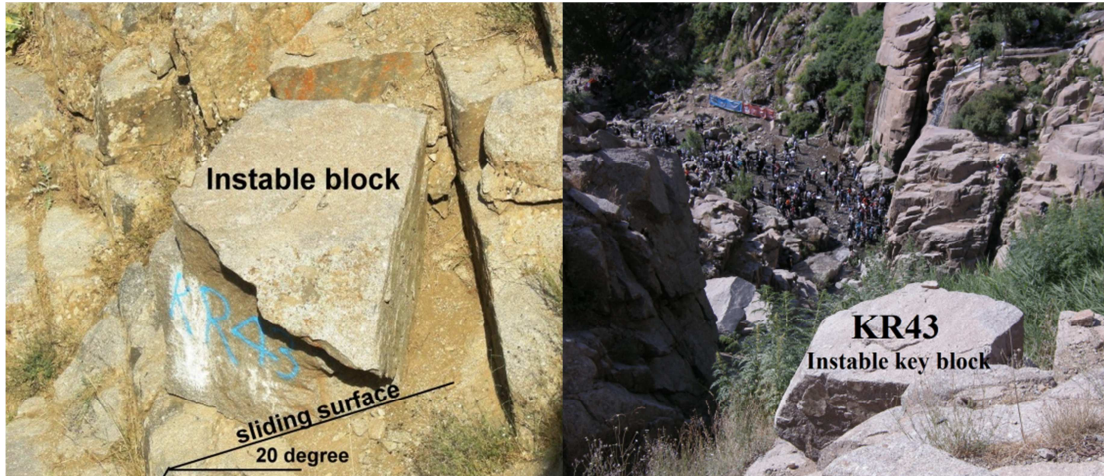
Fig. 6: A view of key block KR43 detaching due to Ice jacking action
