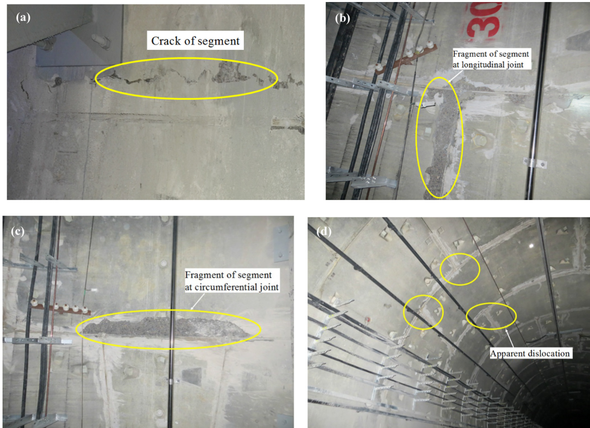
Fig. 7. Typical structural problems observed within the tunnel segments following the application of secondary grouting: (a) Crack within a segment, (b) Fragment of segment at a longitudinal joint, (c) Fragment of segment at a circumferential joint, (d) Apparent dislocation between segments.
