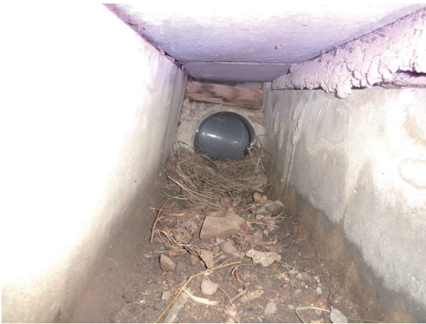
Fig. 3. In a rainwater drainage ditch, over which a few soldierflies were found hovering around openings, there was no trace of the animal's feces but dry grasses used by it for resting on the ditch floor (7 October 2015).
