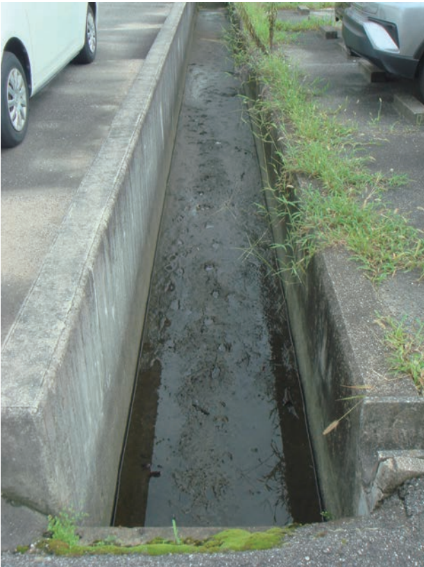
Fig. 3. Footprints on the mud in a ditch between houses (July 16).
