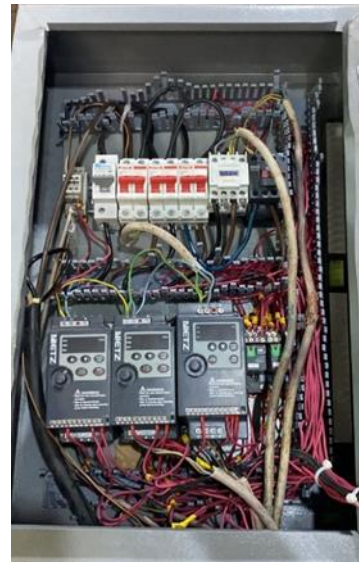
Figure 22: Control Panel Components.
