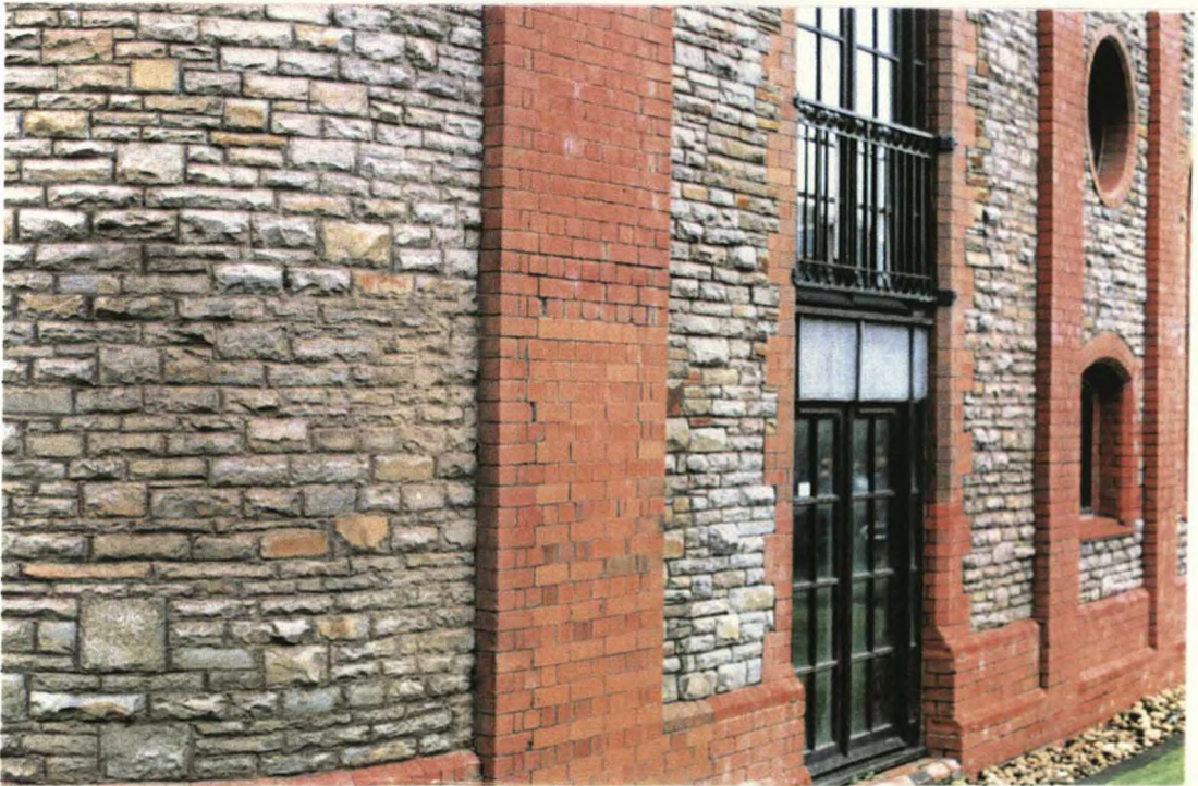
PLATE 4(12). Spillers and Bakers warehouse, Atlantic Wharf, Cardiff, showing brick bands (photograph, the author, 1992)
