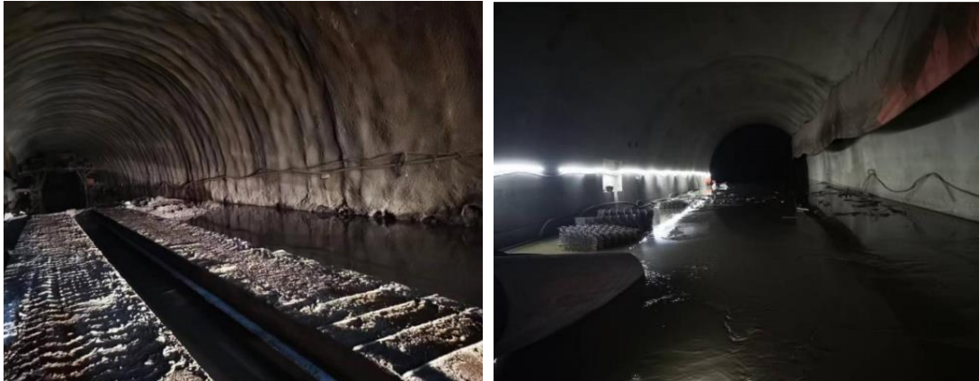
Figure 1. Water Gushing Condition at Site
