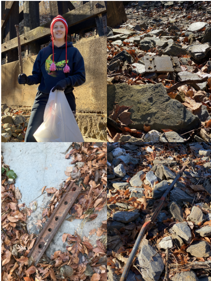
Figure 10. Examples of debris assumed to have come from the railroad above. The items were extremely heavy and showed signs of rust.
