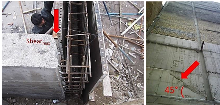
Fig. 3. Wrong construction joint position at a concrete wall joint (left) and a shear wall (right)
