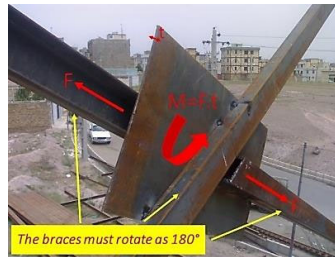
Fig. 8. An example of structural issues due to construction errors in the bracing system
