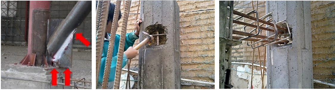
Fig. 7. A weak welded connection of tubular members (left) and a wrong concrete connection (middle and right)
