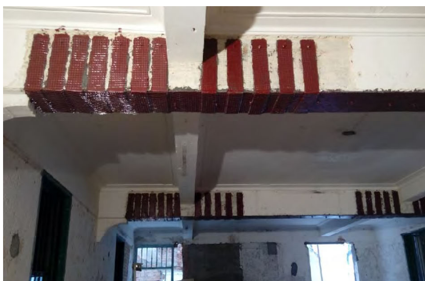
Figure 6.11 Reinforcement added to strengthen an existing floor structure of a pre-1949 building in Shekki, Zhongshan. (Photo by LIU Jianneng, 2015.)
