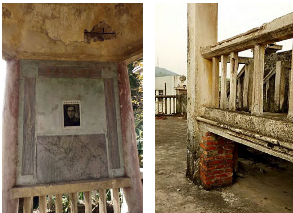
Figure 7.12 On the left, the concrete ceiling of the David O’Young memorial structure in Dai Leng village is spalling and the rusted steel-reinforcement is exposed. (Photo by Christopher Cheng, 26 December 2017.) On the right, the concrete balustrade and rail of the small cupola on top of Cho Bin School in Zhongshan is likewise affected by weathering. (Photo by Christopher Cheng, 7 January 2019.)
