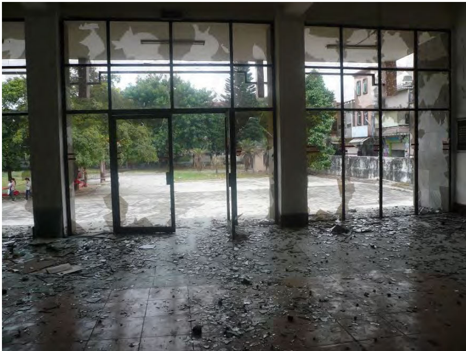
Figure 6.1 The entrance to the library of On Tong School in Dachong, Zhongshan, damaged by vandals. (Photo by Douglas Lam, 2013.)
