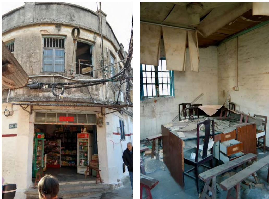
Figure 3.6 A communal hall and minban school built in the 1970s in Duntou village (敦陶村), Shaxi township, Zhongshan. Now it is in a state of disrepair, awaiting demolition. (Photo by Denis Byrne, 21 December 2017.)
