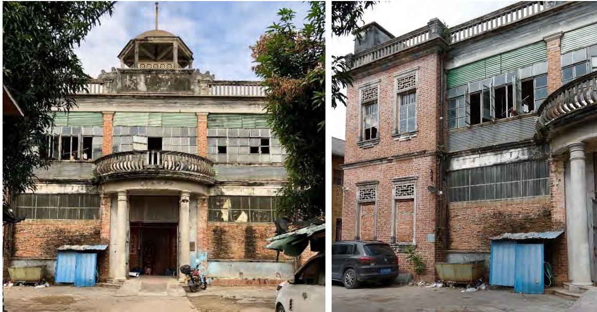
Figure 6.12 The former Sha Chung School in a dilapidated state in 2018. Notice the portico-balcony has been infilled. (Photo by Denis Byrne, 2 December 2018.)
