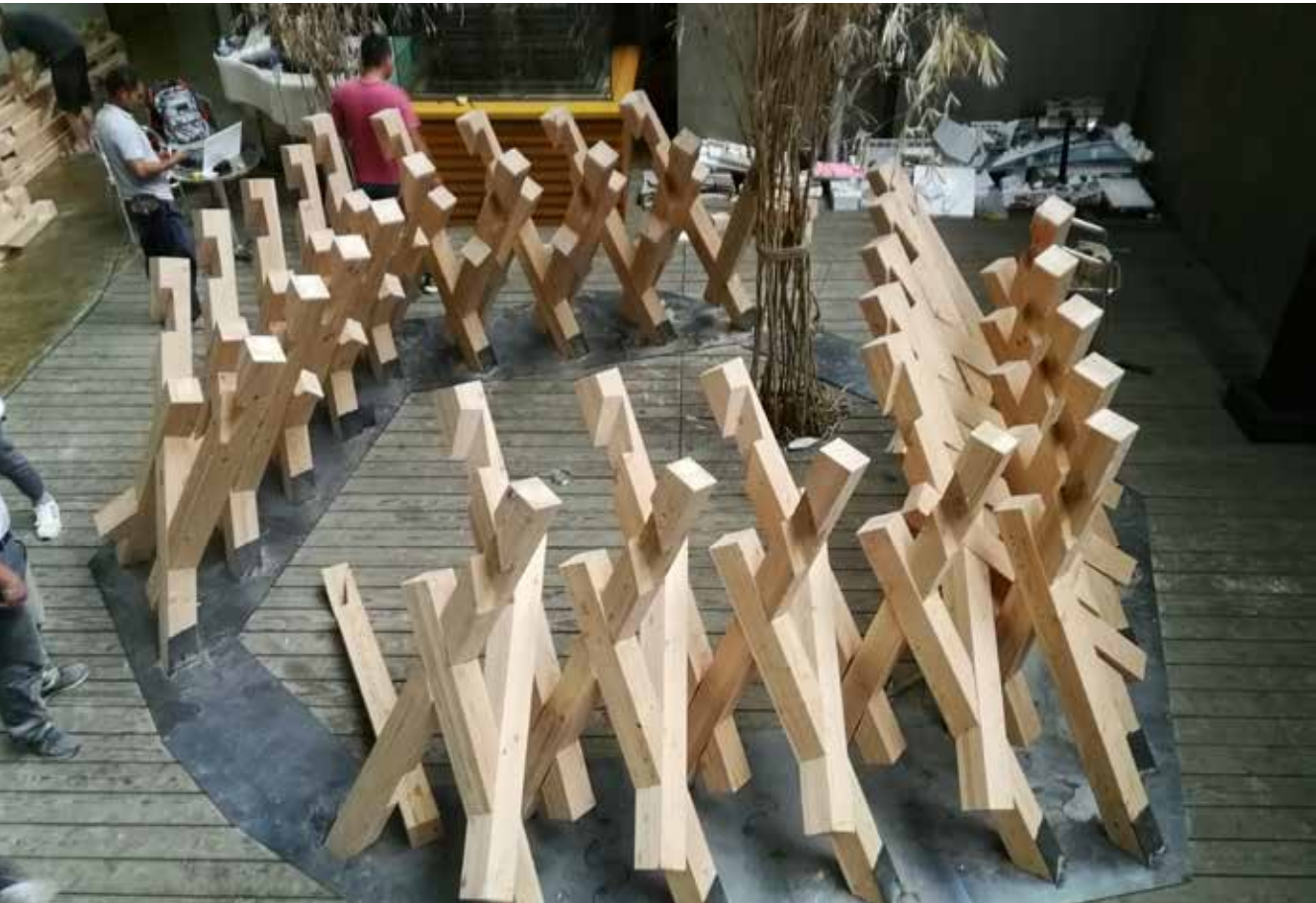
Fig. 6.16 Construction process of the tower on site (hall of the building C at CAUP, Tongji University Shanghai)
