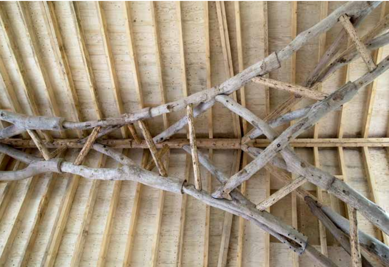
Fig. 5.40 View of the roof truss arch for the Woodchip Barn project in Hooke Park
