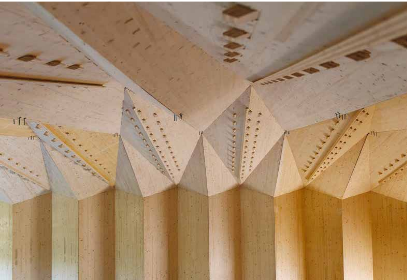
Fig. 3.7 The theater designed by the IBOIS research center of EPFL, Losanne, is an example of ‘fabricated materiality’ that links together the structural principle and the fabrication method.
