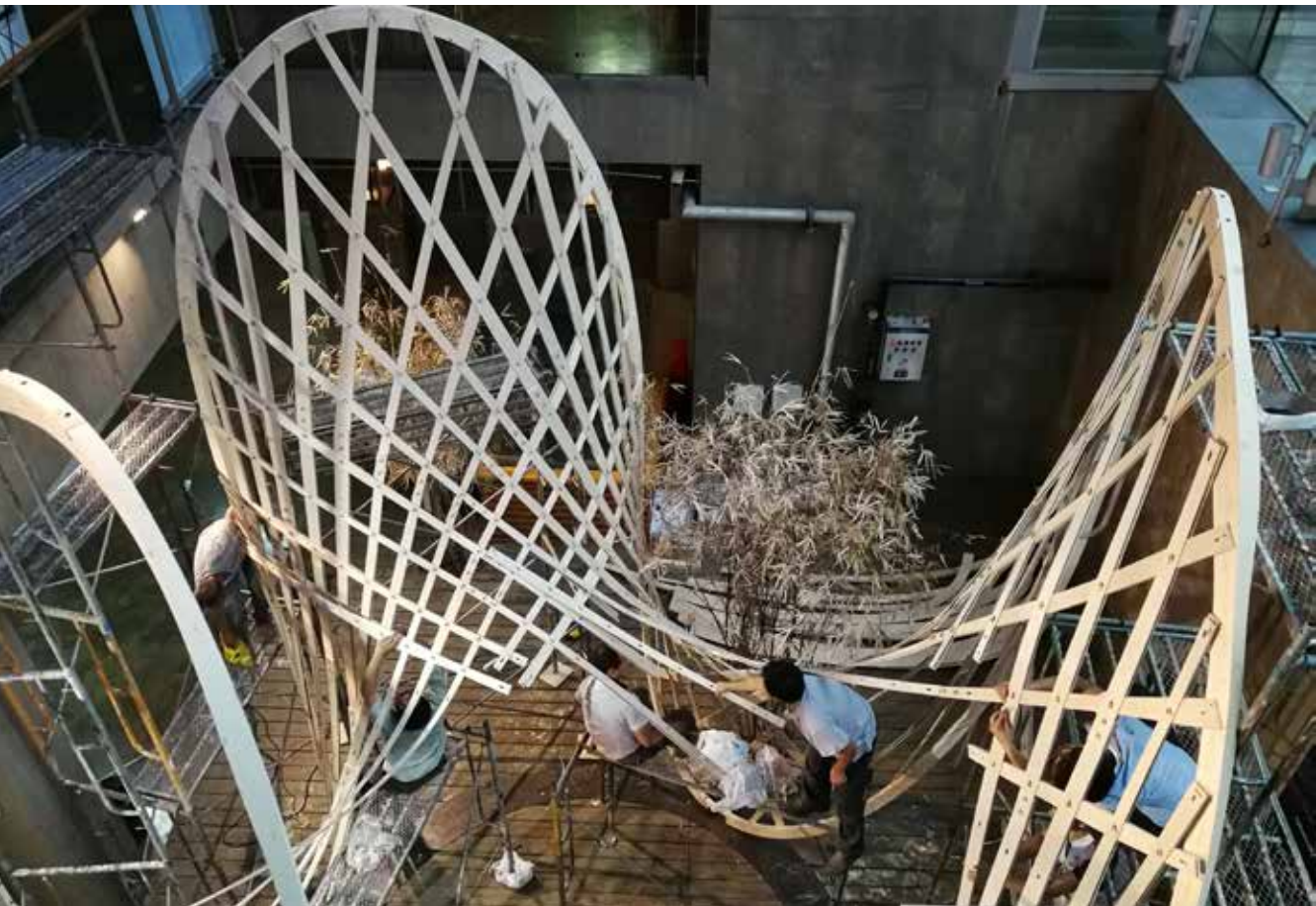
Fig. 6.14 Construction phase of the pavilion on site (hall of building C, in CAUP, Tongji University Shanghai)
