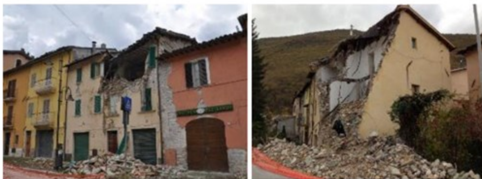
Figure 7.1 Examples of local out-of-plane seismic damage to buildings, observed after the Central Italy sequence of 2016-2017 (Photos: A. Penna – adapted from (Penna et al. 2022))
