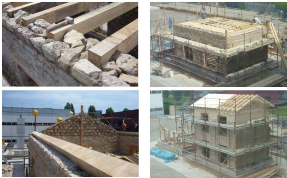
Figure 7.14 Building 1 construction phases: floor and roof connections (left) and diaphragms construction (right) (Magenes et al. 2010a)
