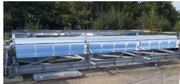
Figure 5: CSP collectors installed in Bochum.
