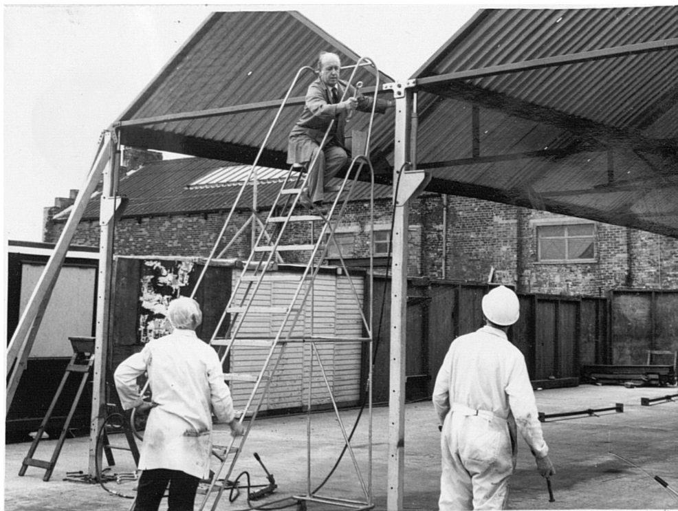
Plate (10.2) Jacking of the roof in stages from moveable knees. External bracing was temporarily attached
