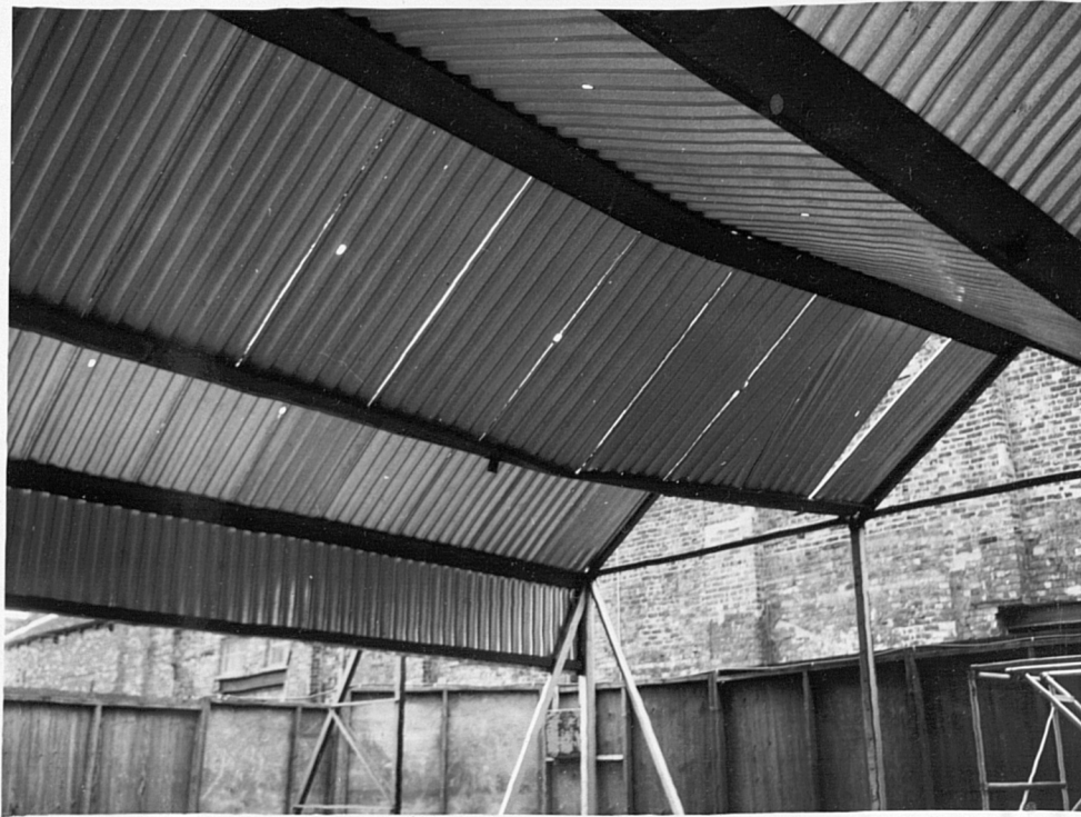
Plate (10.5) Failure occurred by seam tearing of the central bay. This caused excessive twisting of the adjoining fold line members
