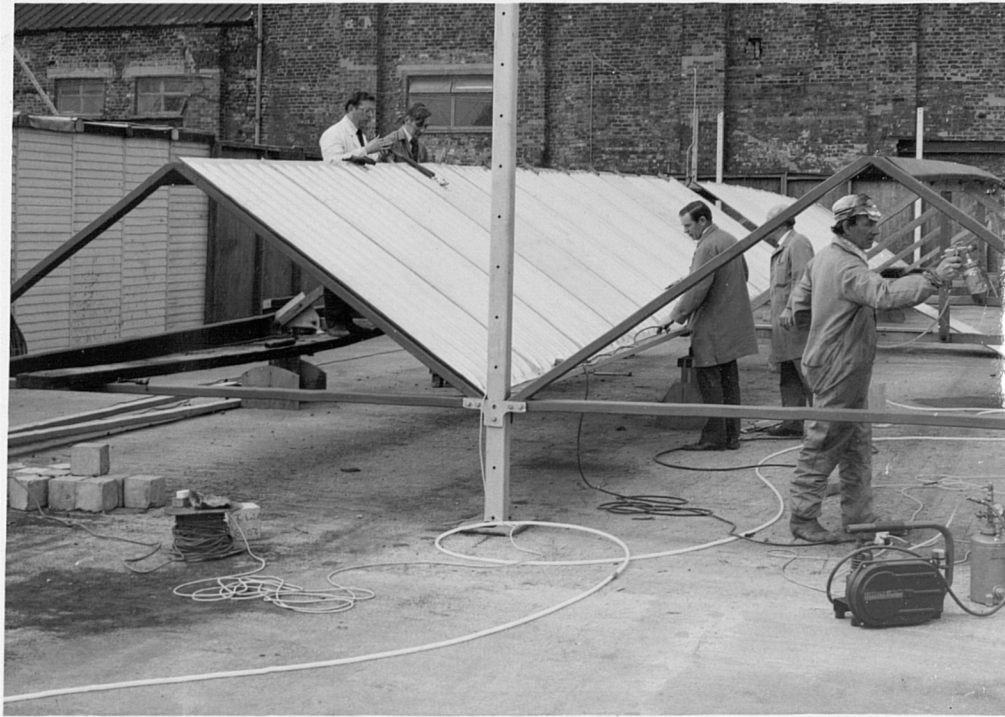
Plate (10.1) Sheeting between fold lines in operation. The fold lines are held in position by wooden trestles which are set to the correct roof camber
