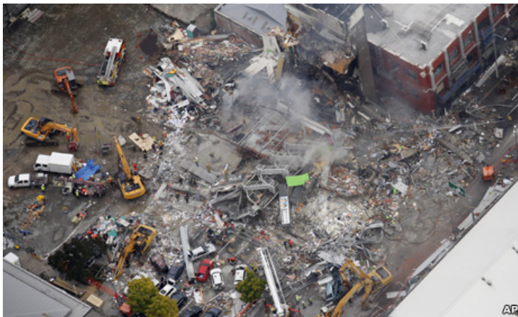
Figure 4-22: CTV Building Total Collapse
