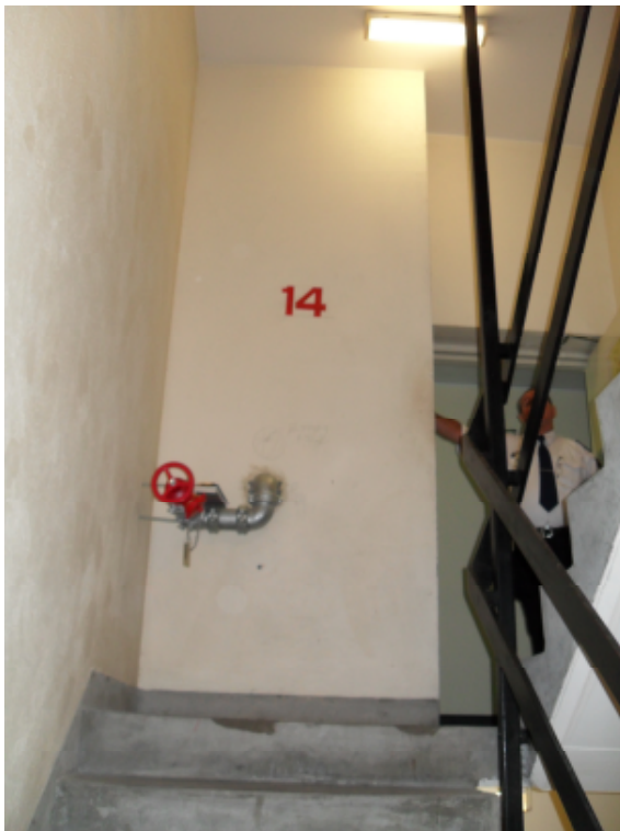
Fig.B3, 8 - Looking up flight from intermediate landing to floor number sign and hydrant valve
