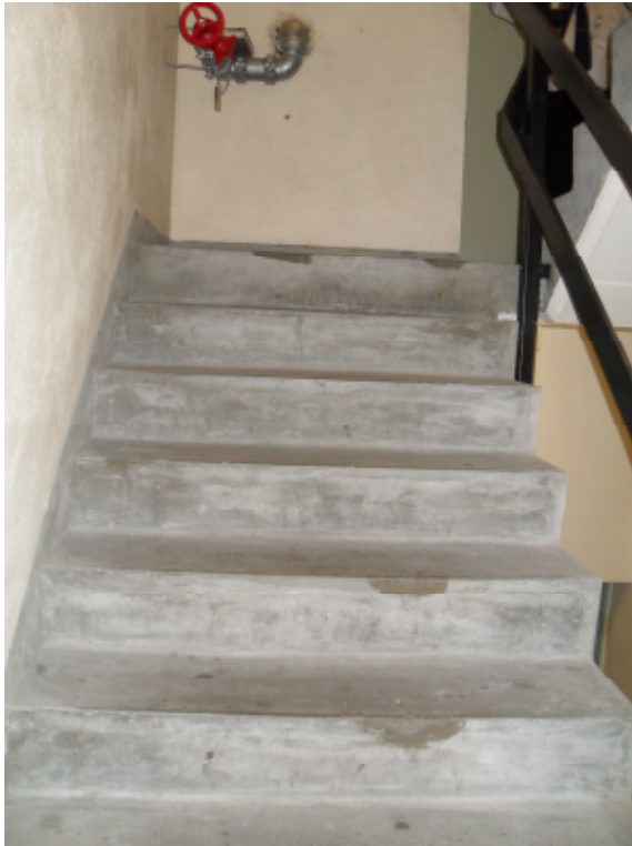
Fig.B3, 9 - Detail of typical steps showing patching
