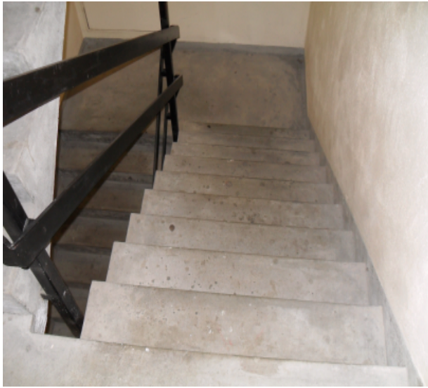
Figure 5-3: Typical example of handrails from Buildings 3 and 7 – rectangular profile and poor graspability.
