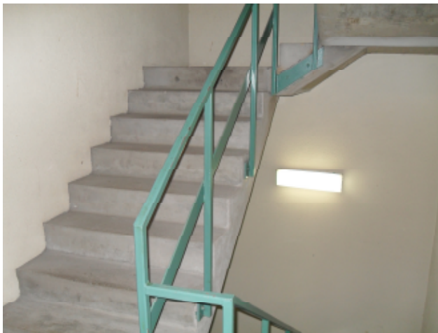
Figure B7.2 - Stair looking up from main landing on Level 10. Note contrasting handrails and emergency lighting on intermediate landing
