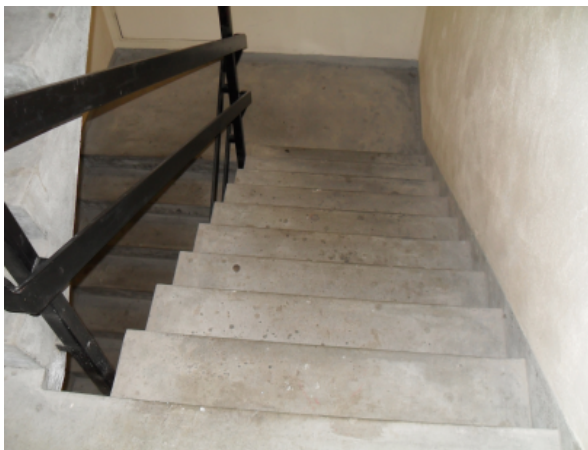
Figure 4-18: Typical View of first stair flight at stair entry – Building 3 – Exploratory Case Study
