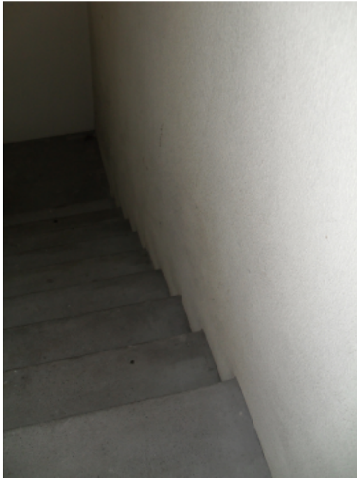
Figure B7.8 - Outline of 'grey' steps against white/ cream wall - note absence of handrail
