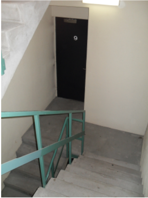
Figure 4-20: Typical view of down flight approaching entry door – Building 7 ( other stair is opposite handed )
