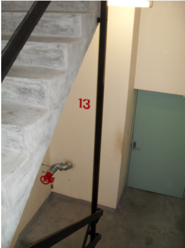
Fig.B3, 7 - Looking across from the intermediate landing to see floor number and hydrant valve
