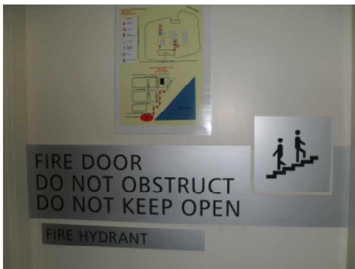
Fig.B3, 2 - Exit access door signage – cluttered
