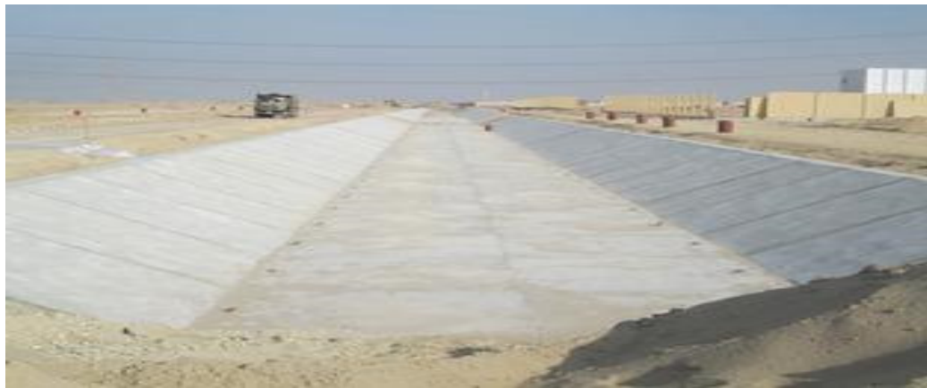
Figure 12.4: Constructed Open Channel in KSA (from the selected ongoing Mega-project, action research)
