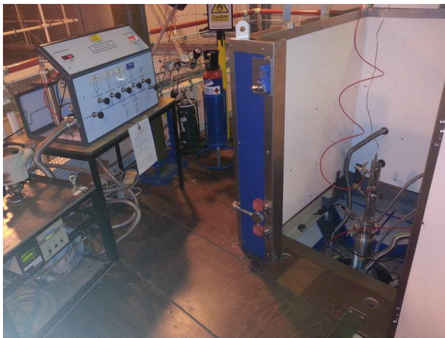
4-C Osiris gas loading equipment
