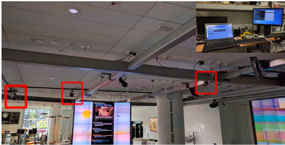
Figure 7.8: The 'egg' suite ceiling infrastructure was designed by the author for the deployment of this and other systems. The Bonita cameras can be seen highlighted.
