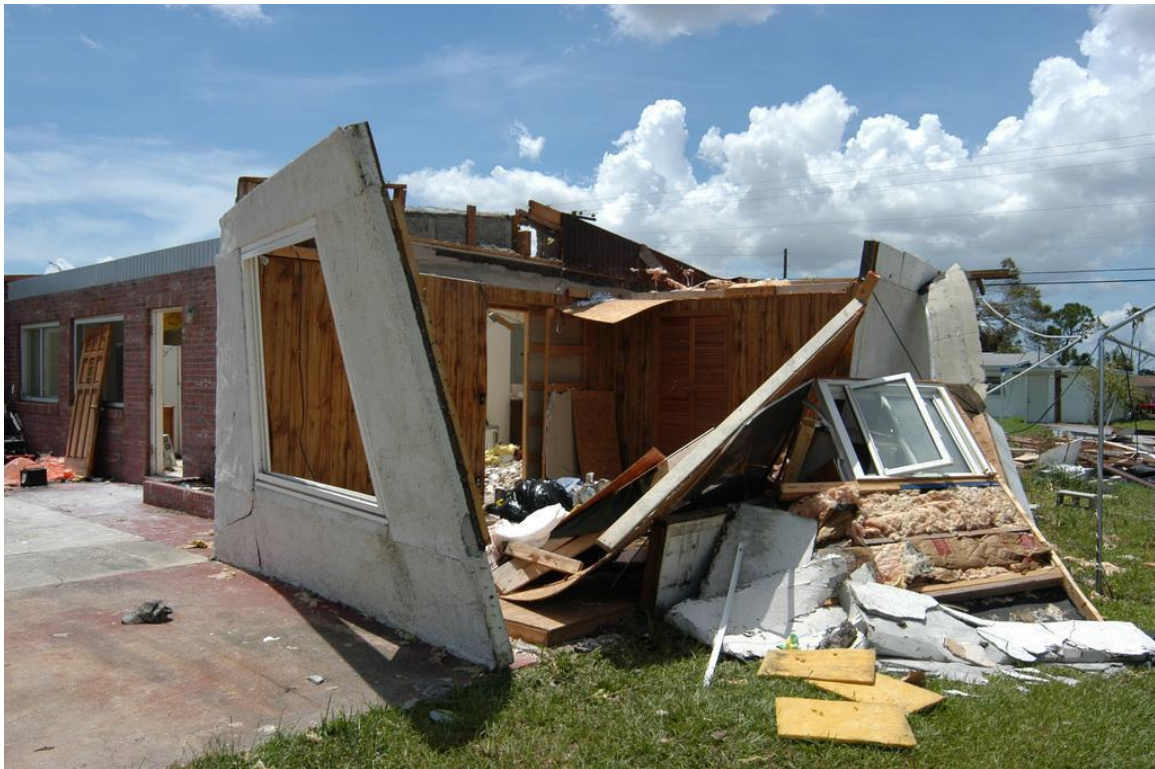
Figure 2.17: Florida – Hurricane Charley Damage, Punta Gorda (Source: FEMA, 2004)
