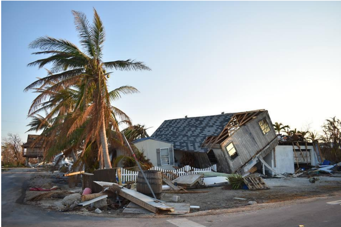
Figure 2.9: Florida – Hurricane Irma Damage, Monroe County (Source: WFSU, 2018)
