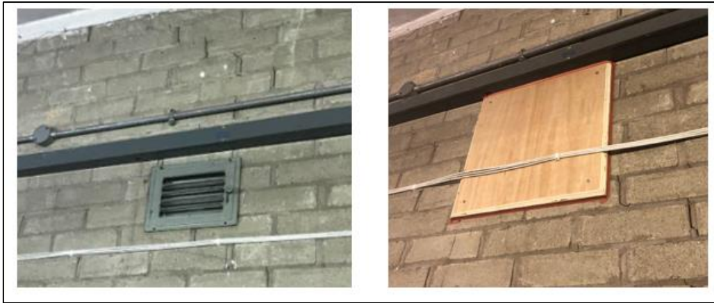
Figure 40: Ventilation Point as Installed (Left) and Blanked (Right)
