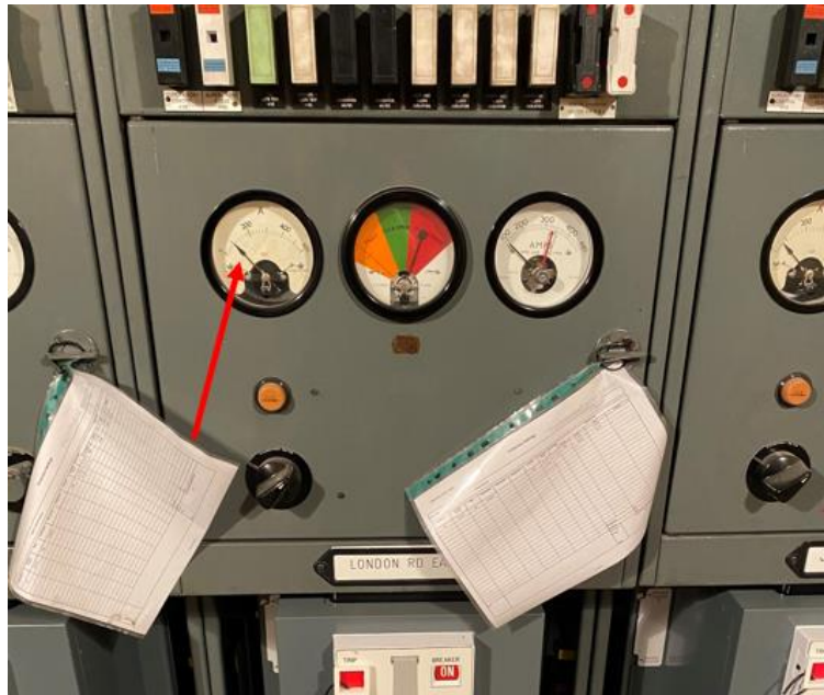
Figure 33: Switchgear Current Reading Dial
