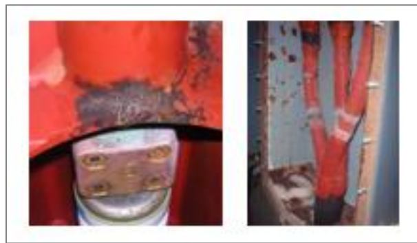
Figure 4: Evidence of PD on Electrical Assets
