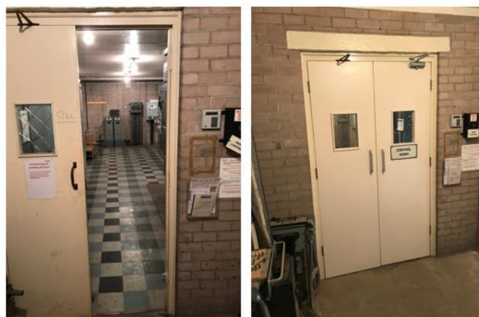
Figure 41: Pendleton Control Room Door Damaged and Repaired
