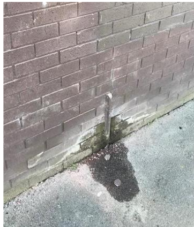
Figure 14: Dehumidifier Drainage Hose Within Substation
