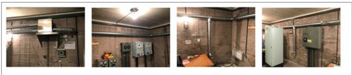
Figure 45: Installed Desiccant Dehumidification System and Ductwork
