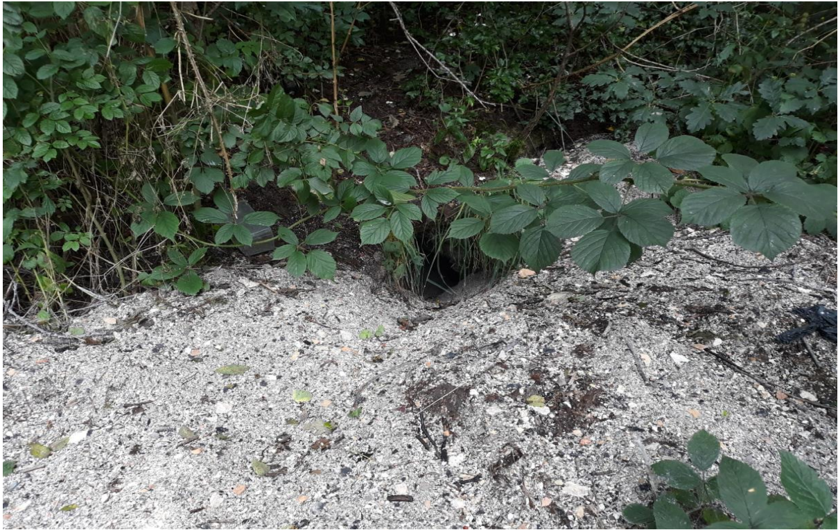
Figure 5.22 Badger sett on the slope bringing white material to the surface
