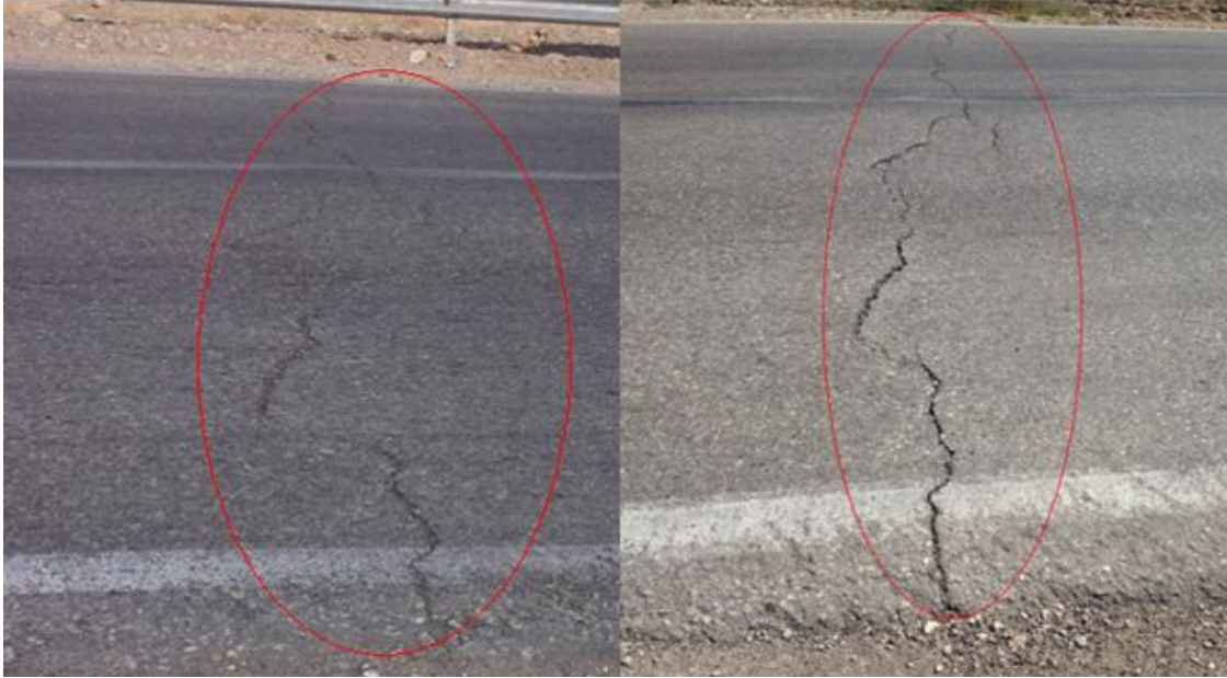
Fig 5. Condition of the cracks in the first observation (2019-12-11)
