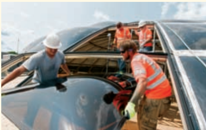
The Koffler Rotunda in the Unistructure underwent major surgery this summer as the 43-year-old acrylic dome panels were replaced. The new panels are thicker, with a dark bronze tint, providing better year-round insulation.
