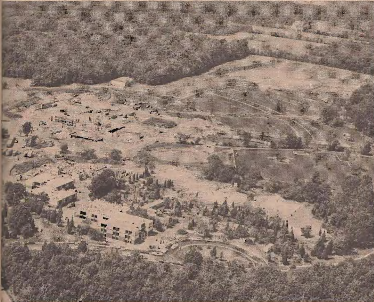
With good fall weather upon us, construction on the new campus is proceeding at a remarkable pace. Many of the planned thirteen dorms are readily recognizable in the foreground. Construction of the "uni-structure" is visible in the left background. The light shaded area in the upper right is the sitework already completed on the gymnasium.
