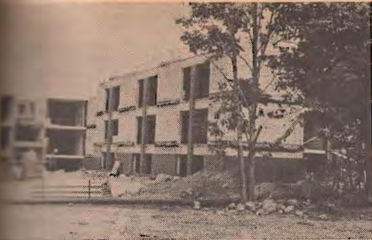
Dormitories on the new campus are said to be ahead of schedule. Above, finishing brick is being placed on one of the buildings. Work is expected to be completed by June 1st.
