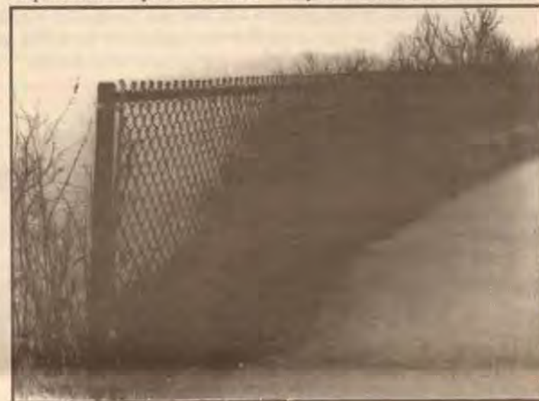
A chain-link fence like this was placed around the area of the Cliff Walk where Michael Cain fell. As you can see by the divot under the fence, the path is worn in certain areas and poses a potential danger to all those who walk the path. The author stood in the divot and without the support of the fence, would have fallen to the rocks below.
