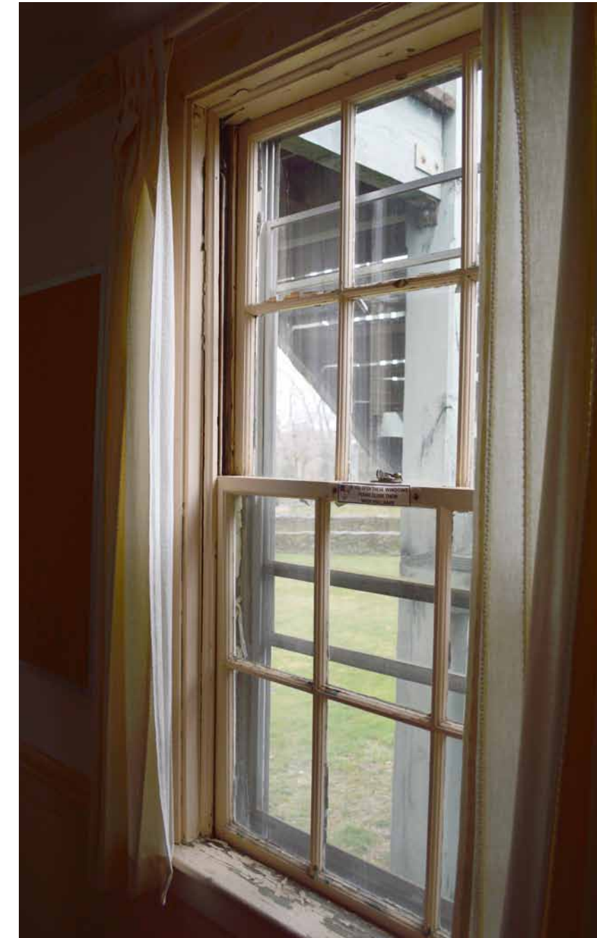
The windows are in varying states of disrepair. Many require repainting and replacement of rotting sills.
