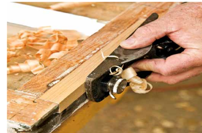
Window repair requires removing hardware, scraping paint by hand and re-glazing the glass.
