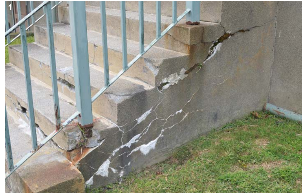
1. The front stairs exhibit significant cracking and loss of concrete. The railings show rust and paint loss.
