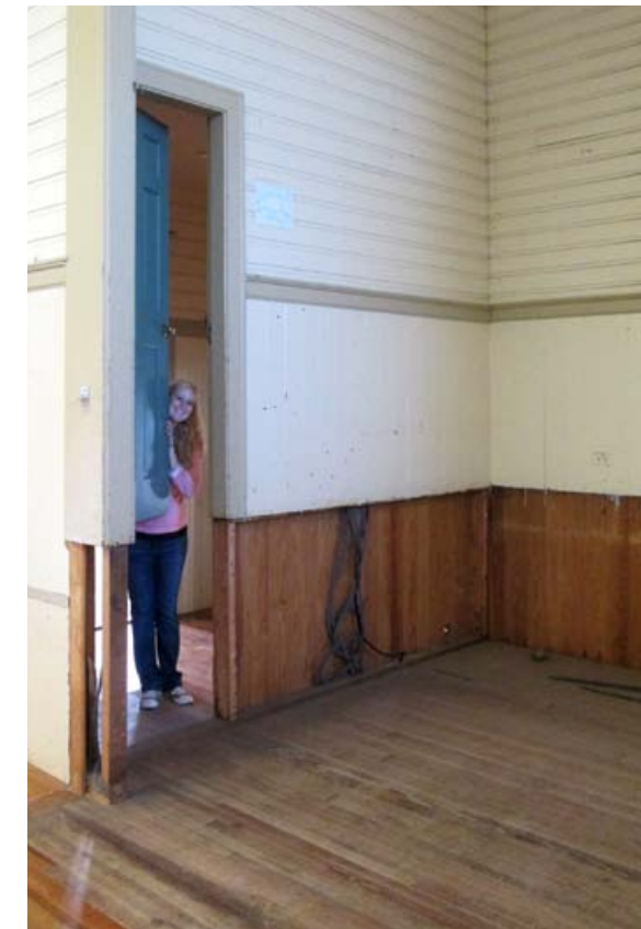
A team member peeks through one of the floating doors of the removed stage area.
