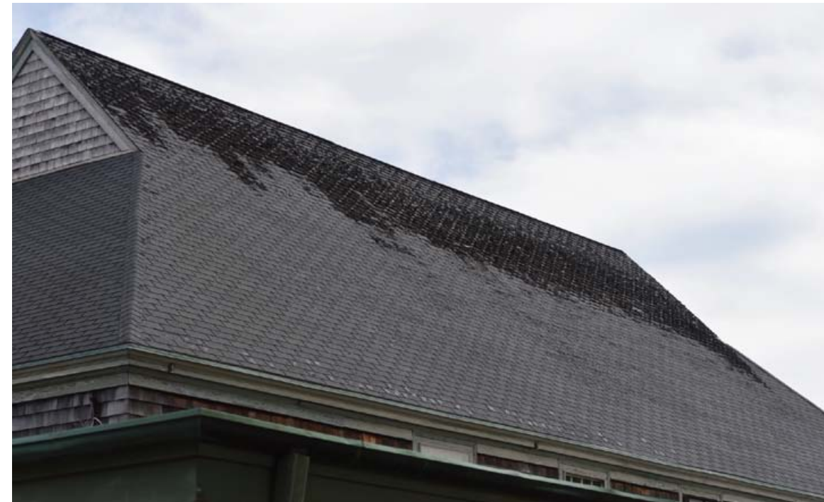
The deteriorating asphalt roof needs to be replaced, potentially with red cedar shingles to achieve historic appearance.
