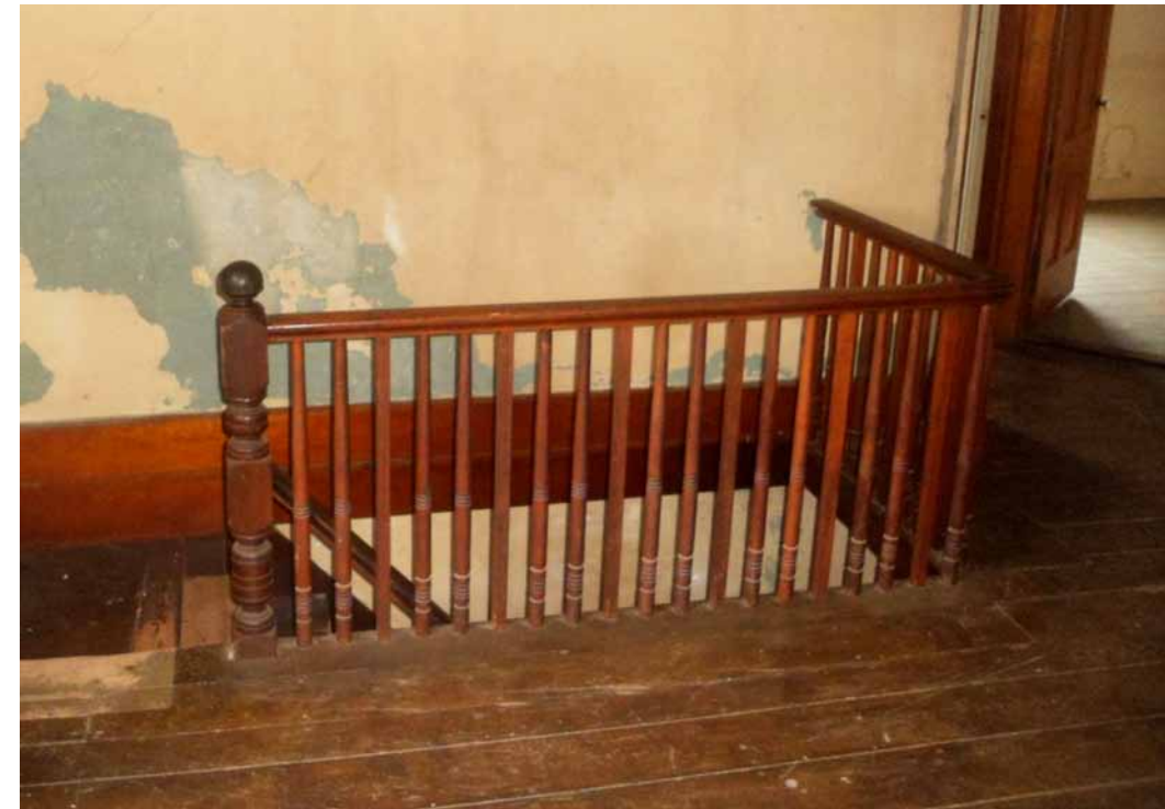
Wood floors and banisters need to be cleaned and refinished.
