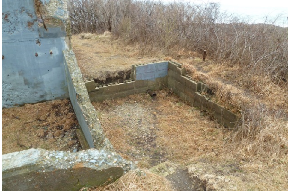
[Fig. 9] View of the latrine foundation walls, looking south. Note the missing CMU blocks.
