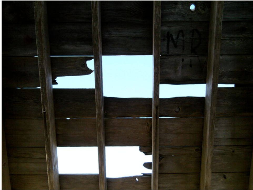
[Fig. 11] Detail of roof holes. The surrounding roof decking remains in good condition.
