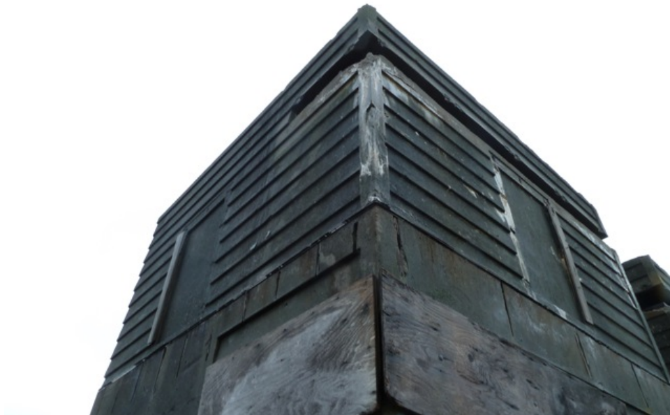
[Fig. 10] Detail of the southwest corner. Note the excessive efflorescence and locations of remaining window jambs bordering each of the two blind windows.
