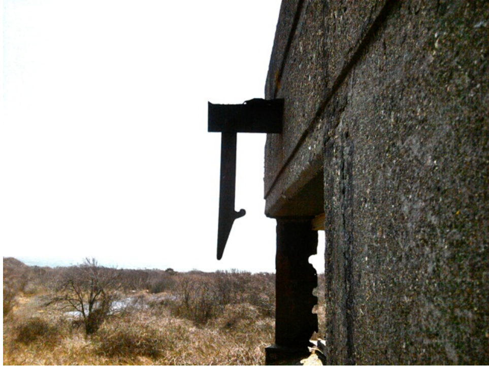
[Fig. 27] View of second story window hook and mount on west elevation, looking south. Note corroded steel corner support.
