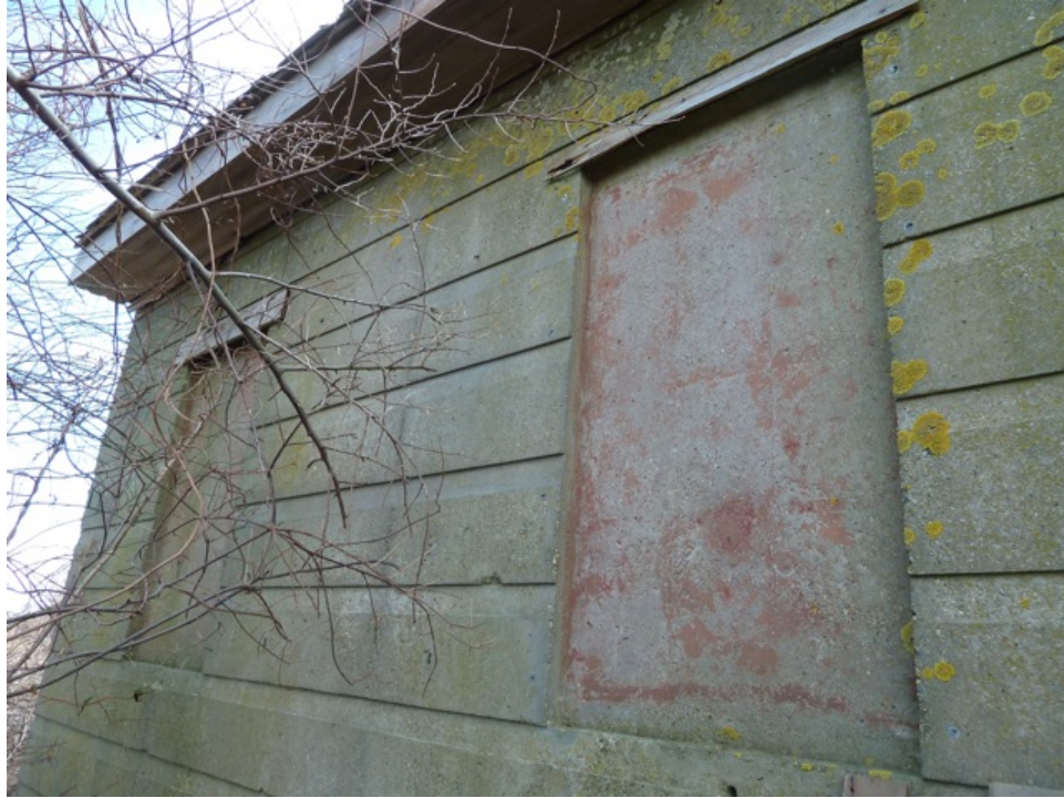
[Fig. 19] Detail of blind windows on north elevation, looking southeast. Note intact wooden lintels, soffit boards, and reddish-brown paint treatment.
