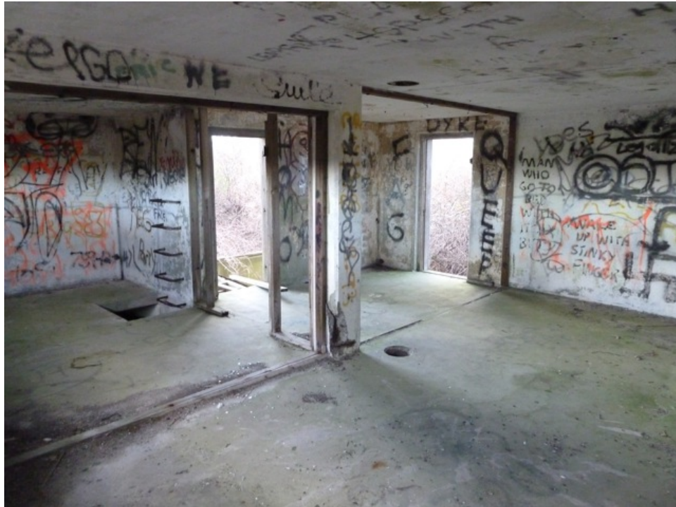
[Fig. 13] View of Room 1-1, looking northwest. Note the wooden framework for partition walls, ladder rungs, and original paint treatment under graffiti.
