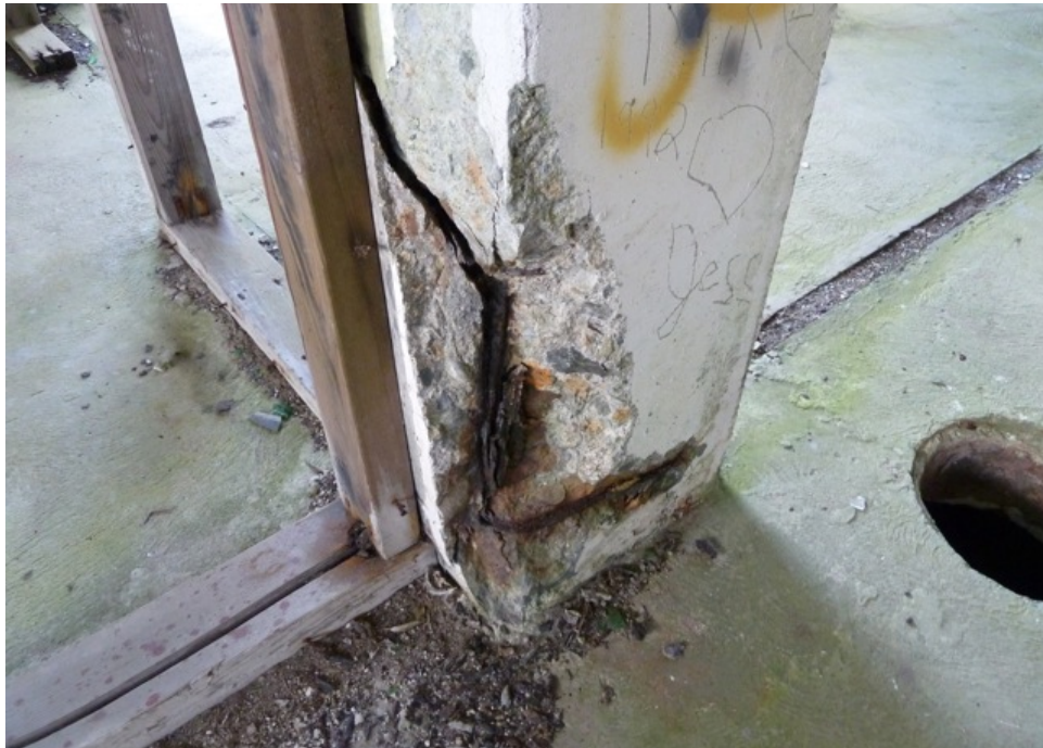
[Fig. 16] Detail of deterioration of central column in Room 1-1, looking northwest. Moisture exposure has led to reinforcement bar corrosion.
