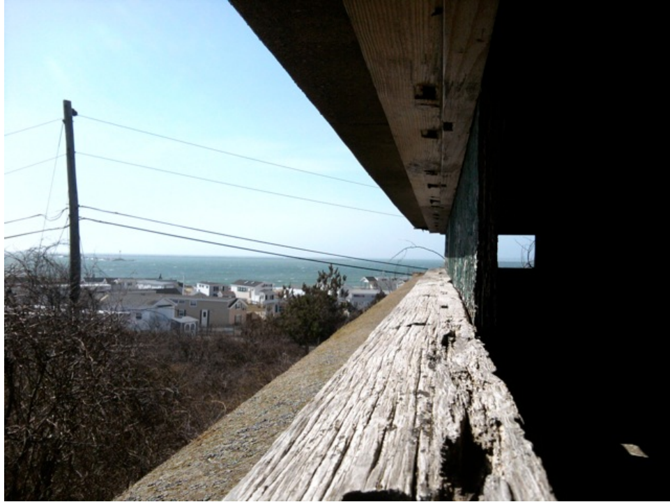
[Fig. 21] Detail of ribbon window frames in Room 2-1. Marks on the upper frame were for the hinges of each awning window.
