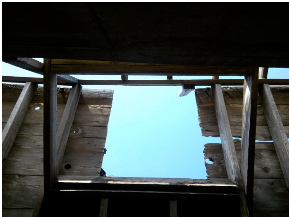
[Fig. 18] Detail of false chimney opening. Note the single remaining 2x4 on the upper right corner. This remnant can be used to attain an accurate height for the reconstructed false chimney.
