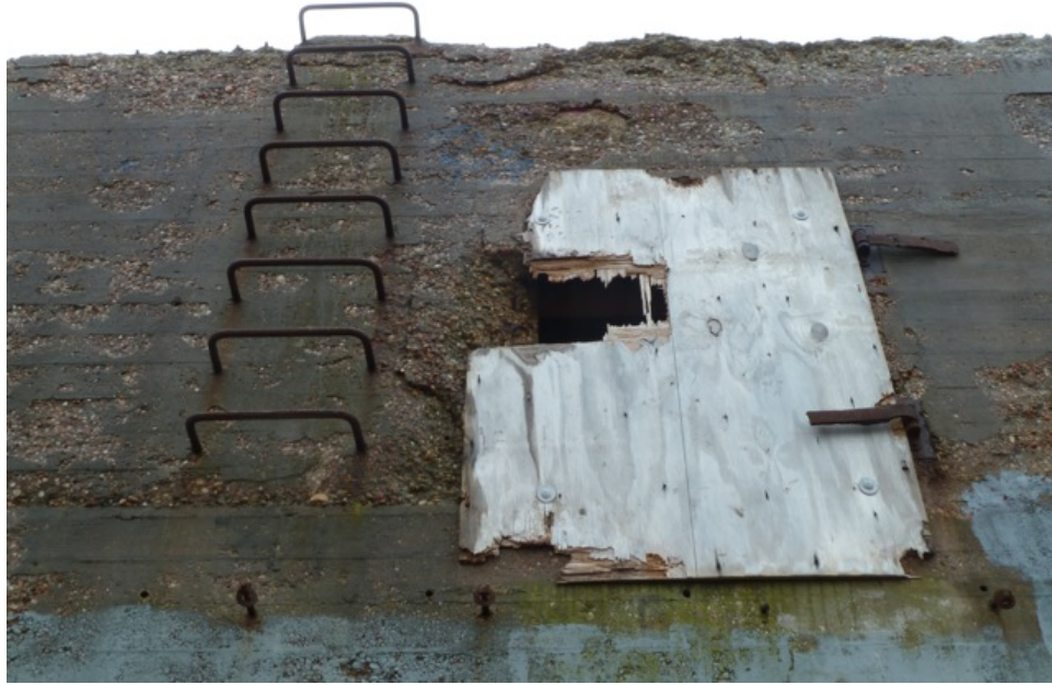
[Fig. 15] Detail of northwest elevation, looking southeast. Note the excessive erosion throughout.
