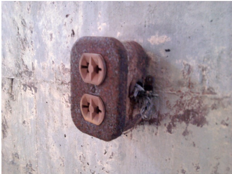
[Fig. 24] Detail of intact electrical outlet.
