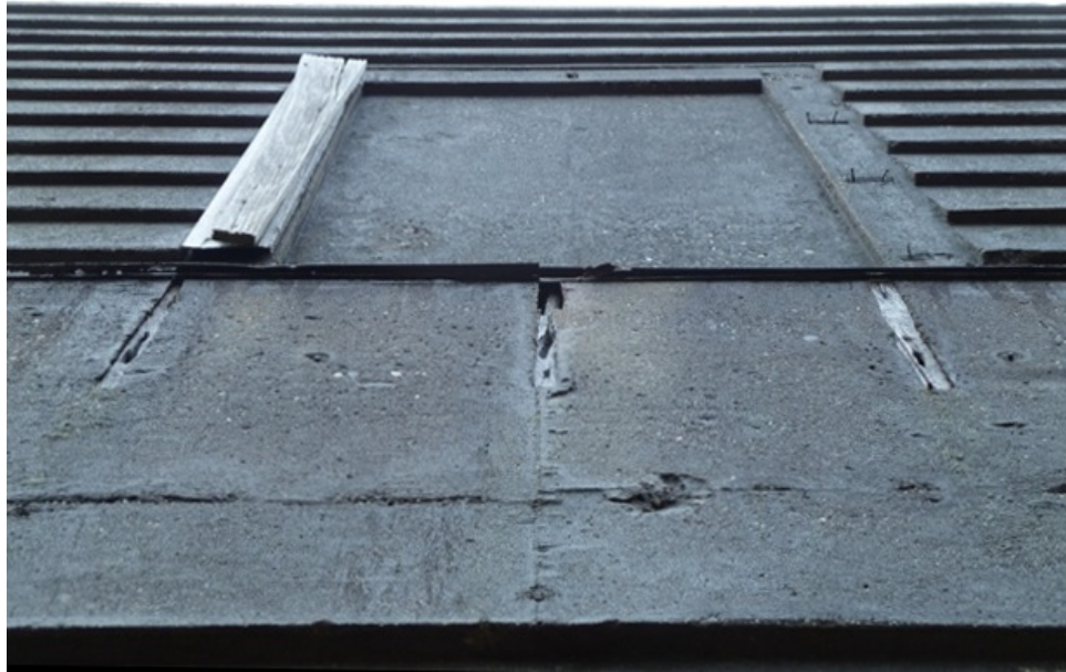
[Fig. 11] Detail of the west elevation. Note the smooth concrete where the porch roof was located, the blind window with associated wooden jamb, and concrete formed to mimic wooden clapboards.
