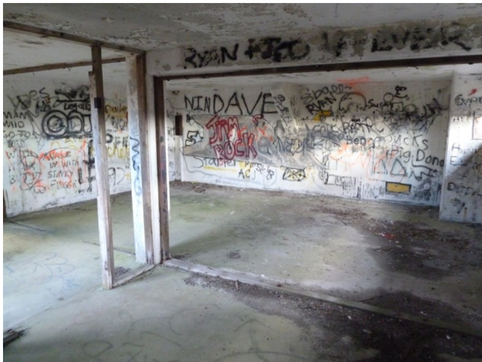
[Fig. 12] View of Room 1-1, looking northeast. Note the wooden framework for partition walls and original paint treatment under graffiti.
