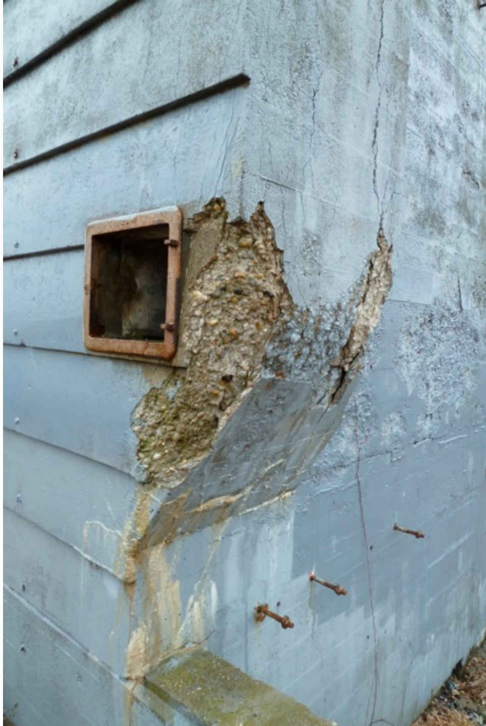
[Fig. 14] Detail of northeast chimney base, looking south. Note excessive erosion and efflorescence, as well as metal doorframe around the chimney access hatch.
