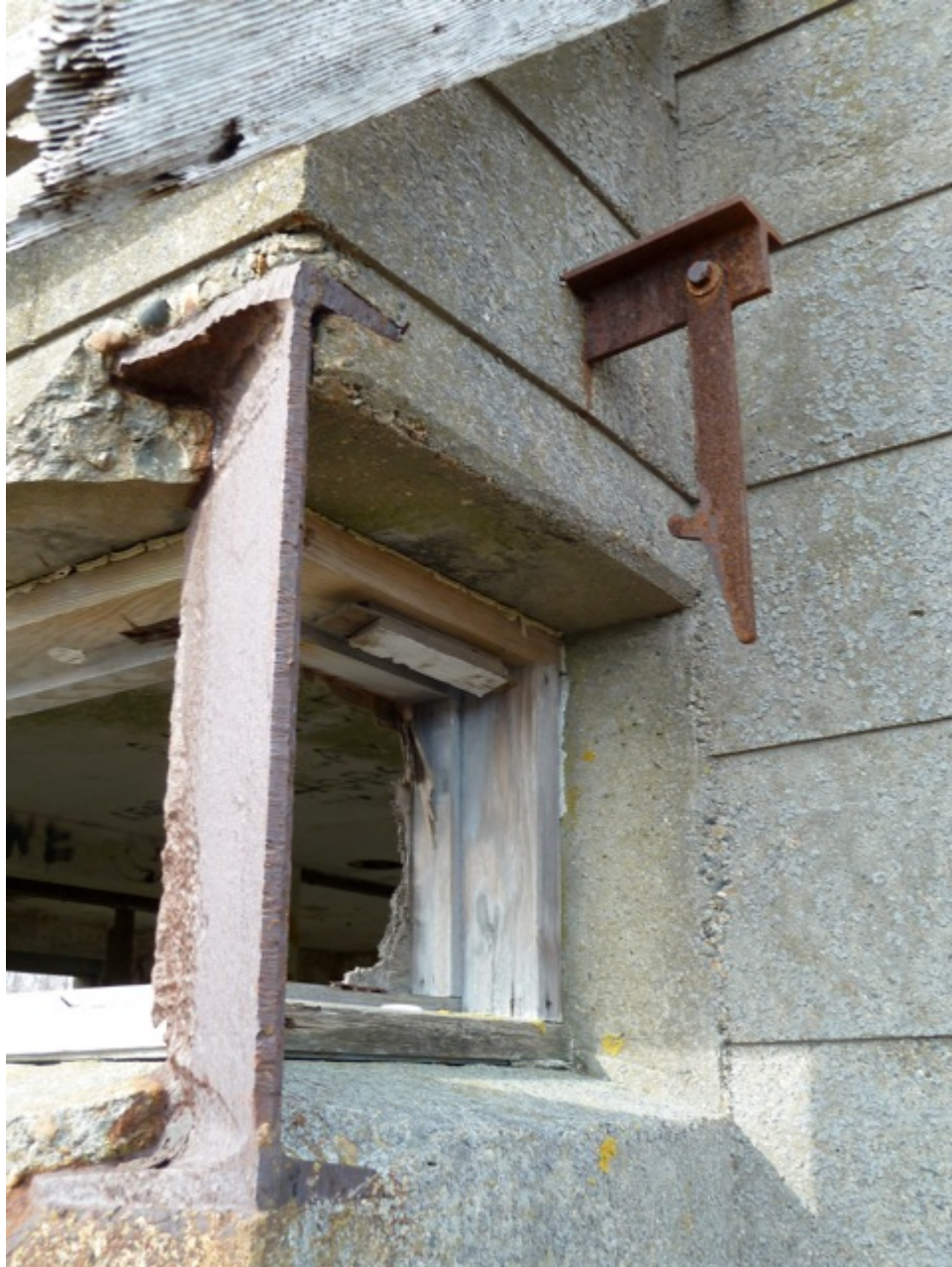
[Fig. 20] Detail of first floor ribbon window, looking northwest. Note the cracked concrete, wooden window frames, remnant of window sash, and intact window hook and mount.
