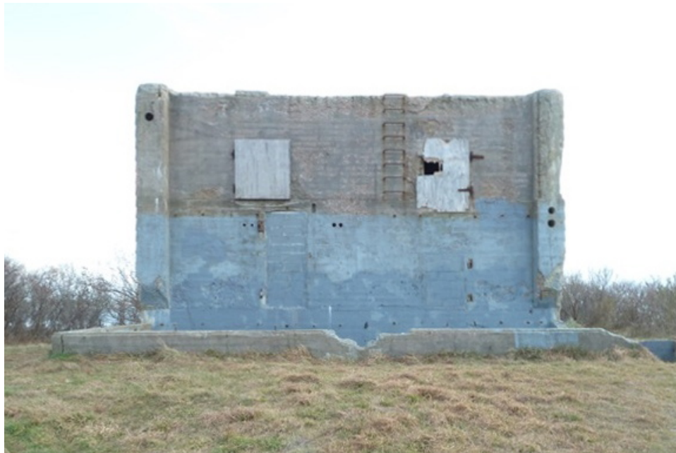
[Fig. 4] View of northwest elevation, looking southeast. Note the exposed ladder rungs and excessive erosion.
