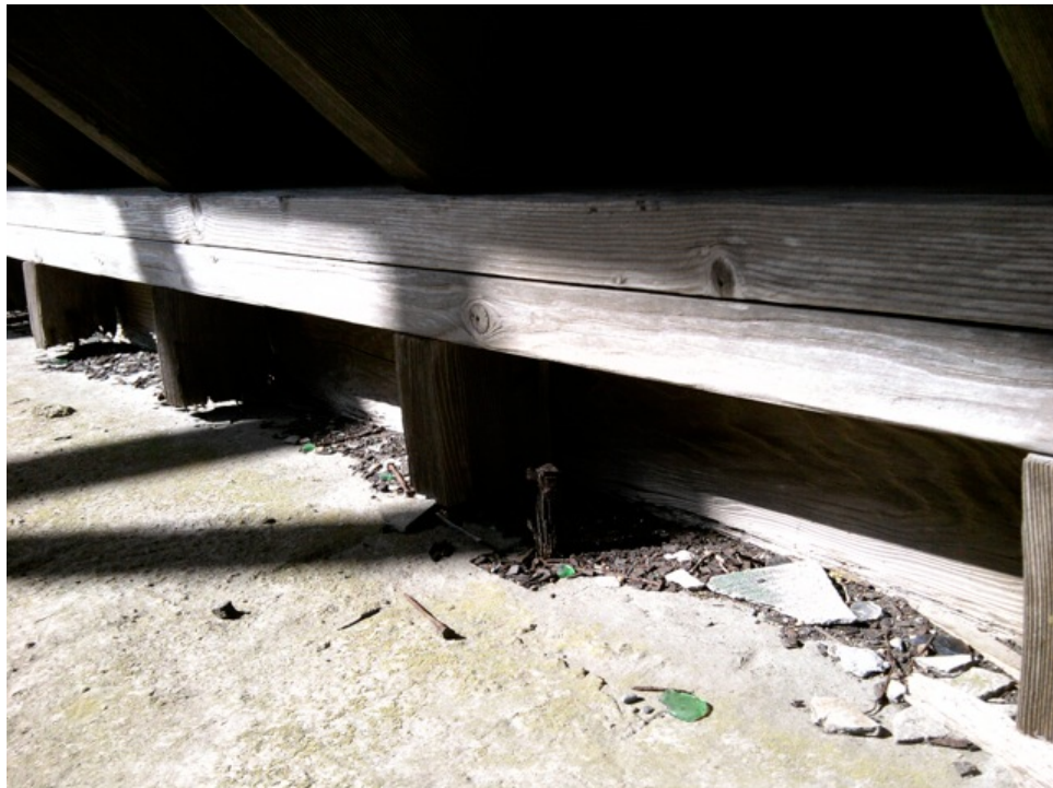
[Fig. 16] Detail of sill plate and roofing system, looking northwest. Note the missing sillplate.
