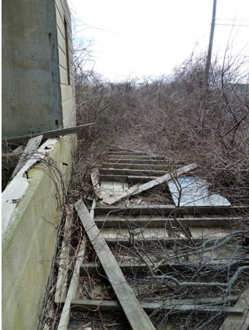
[Fig. 28] Fallen wooden wall for west elevation, looking south.
