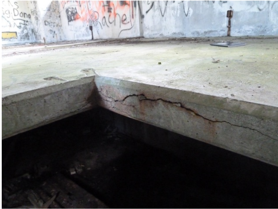
[Fig. 15] The cracking suggests delamination has occurred due to moisture infiltration. Note electrical outlet boxes on the south wall.
