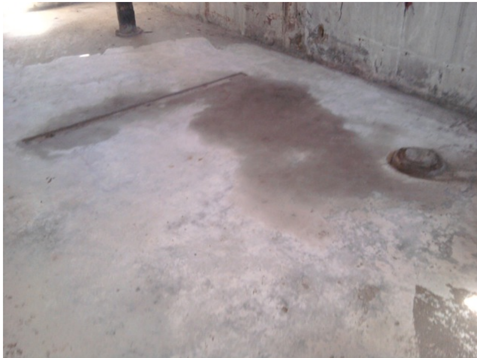
[Fig. 22] View of the floor in Room 2-1, looking southeast. Note the base of a second scope mount in addition to the one in extant.
