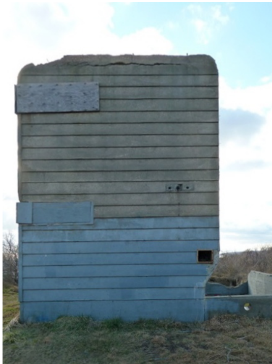
[Fig. 6] View of the northeast elevation, looking northwest. Note the excessive erosion and cracking at the roofline.
