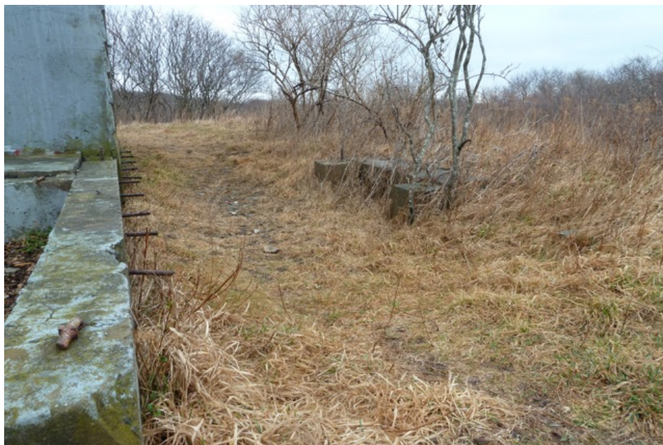
[Fig. 8] Detail of attached porch location, looking south. Note the numerous steel ties and concrete pylons west of the main structure.
