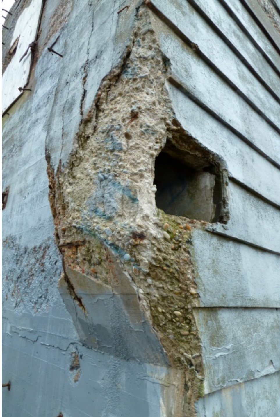
[Fig. 13] Detail of the southwest chimney base, looking east. Note the excessive erosion led to exposed reinforcement bars.
