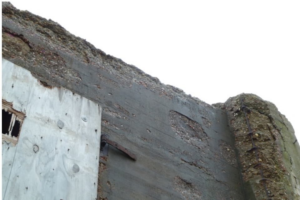
[Fig. 16] Detail of northwest elevation, looking south. Note the excessive erosion and exposed reinforcement bars at the top of the southwest chimney base.
