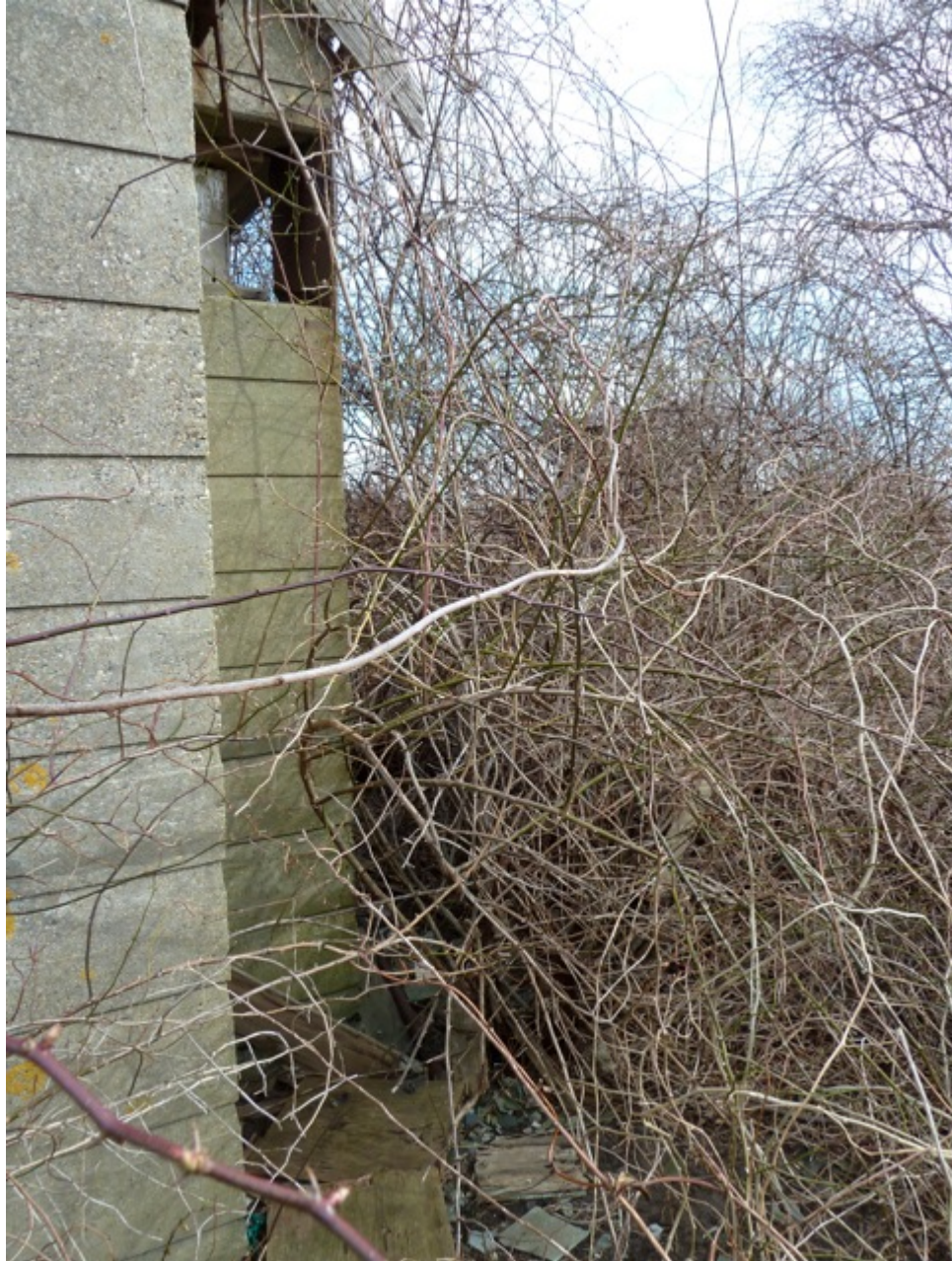
[Fig. 26] View of southwest recessed corner, looking southeast. Note the dense overgrowth.
