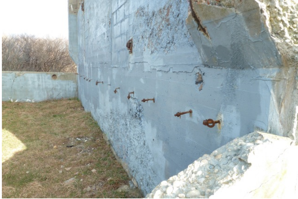
[Fig. 12] Detail of northwest elevation, looking east. Note the numerous steel ties suggesting the location of the now missing wooden floorlevel.
