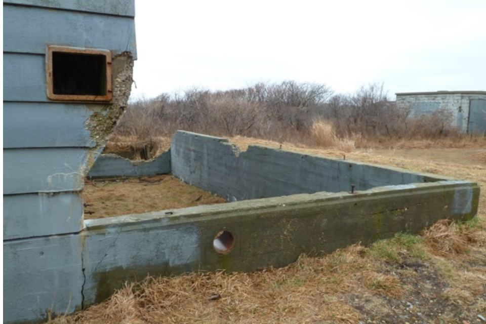
[Fig. 7] View of the foundation, looking west. Note the west generator building in the background.
