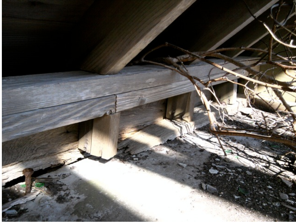
[Fig. 17] Detail of sill plate and roofing system, looking northeast. Note increased deterioration of wood and steel members.
