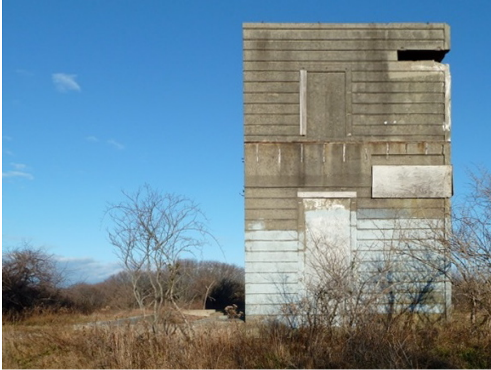
[Fig. 5] West elevation, looking east. Note the remaining door lintel and window jamb.
