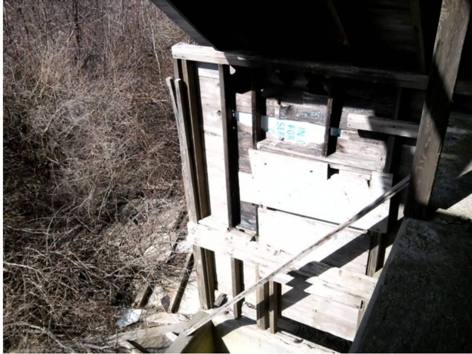
[Fig. 7] View of wooden portion of north elevation. Note the traces of a small fire to the left of the window.
