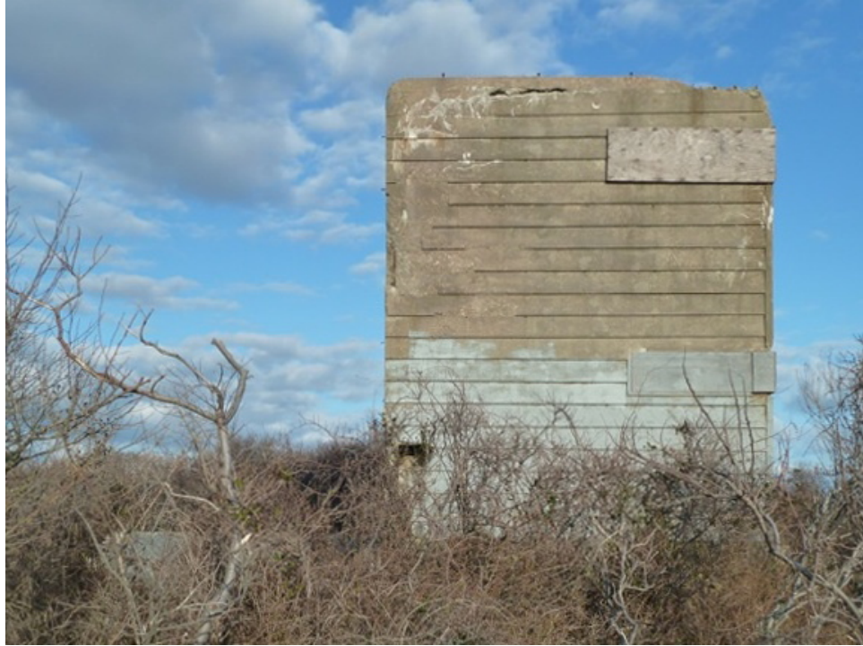
[Fig. 5] View of the southwest elevation, looking southeast. Note the excessive erosion and efflorescence.
