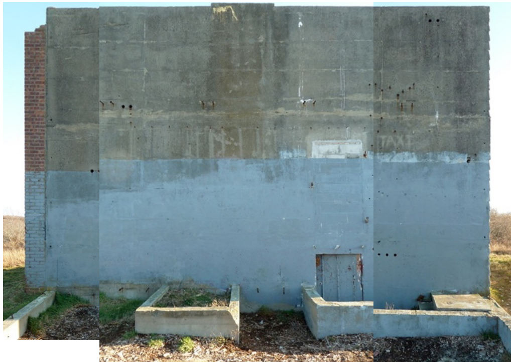
[Fig. 4] Collage of north elevation, looking south. Note the split-level transition between the concrete and foundation levels.
