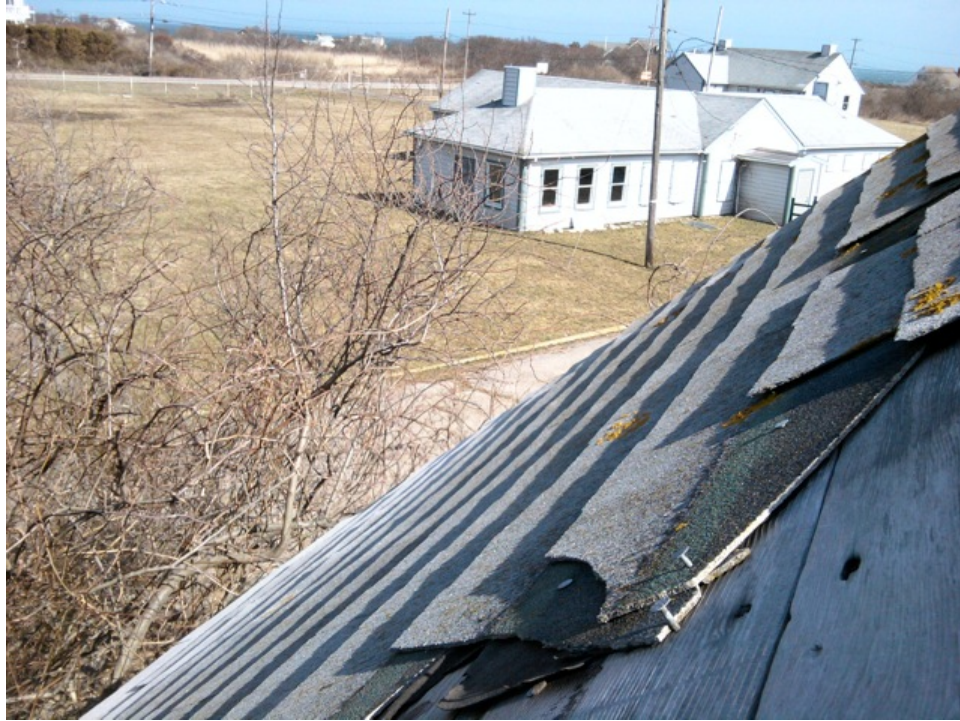
[Fig. 9] View of asbestos shingle roof, looking northeast. Note the two additional buildings on the property. Both were support buildings for Station 1-B and the other two FC stations, Station 1-C and 2-C, within the south reservation. The two stations were torn down in the latter part of the 20 th century. 163
