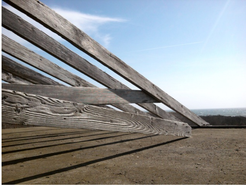
[Fig. 13] Detail of roof structure, facing southeast. Although weathered from exposure, the rafters have remained in good condition.
