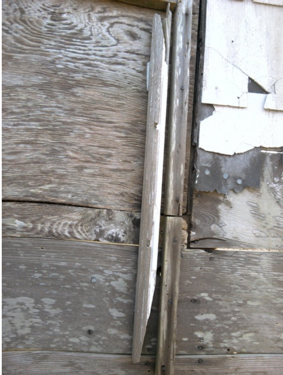
[Fig. 22] View of ribbon window sash remnant on the north elevation, looking south. The remnant is painted white and reused for bracing plywood covering the stair hall window opening.
