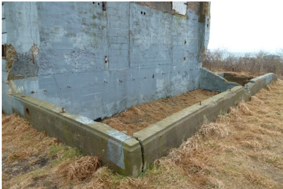
[Fig. 8] View of the foundation, looking south. Note the large crack where the southeast and northeast foundations walls meet.
