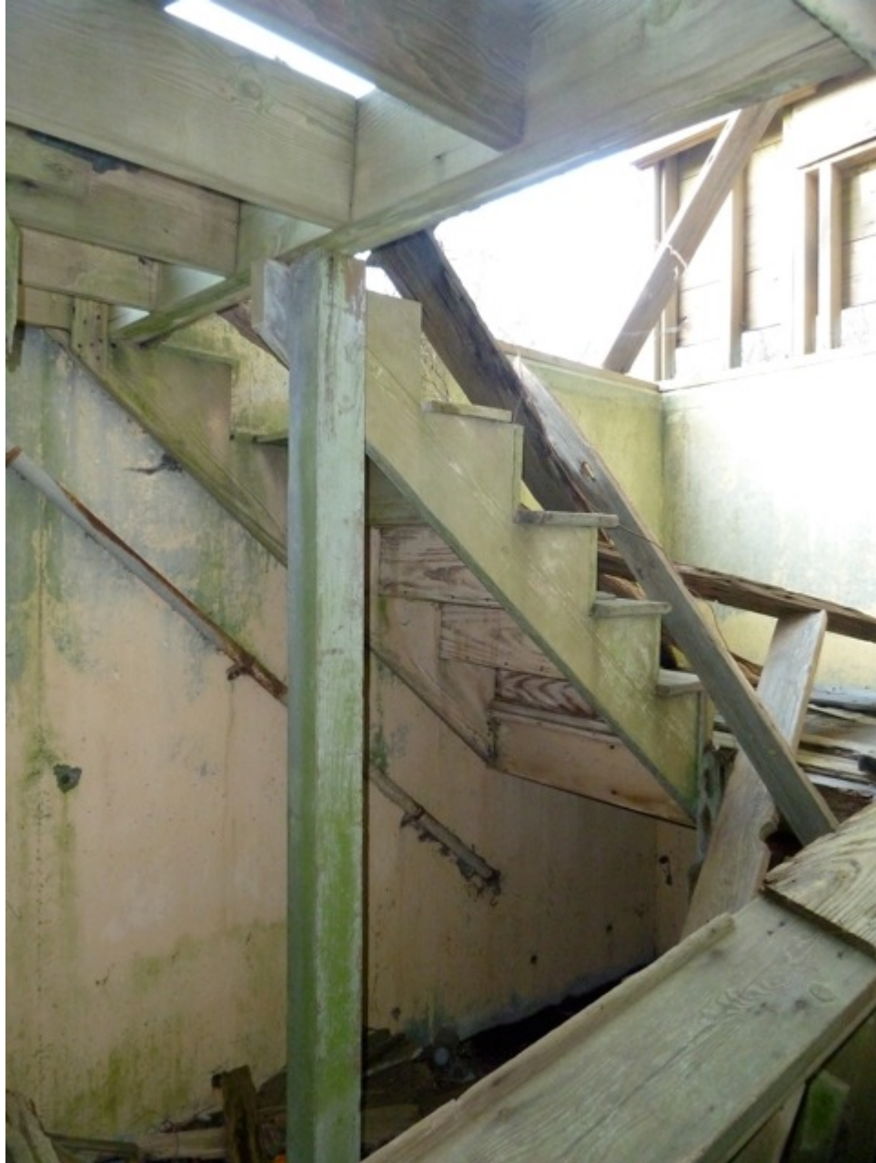
[Fig. 6] View of the stair hall, looking northwest. Note original stair configuration and condition.
