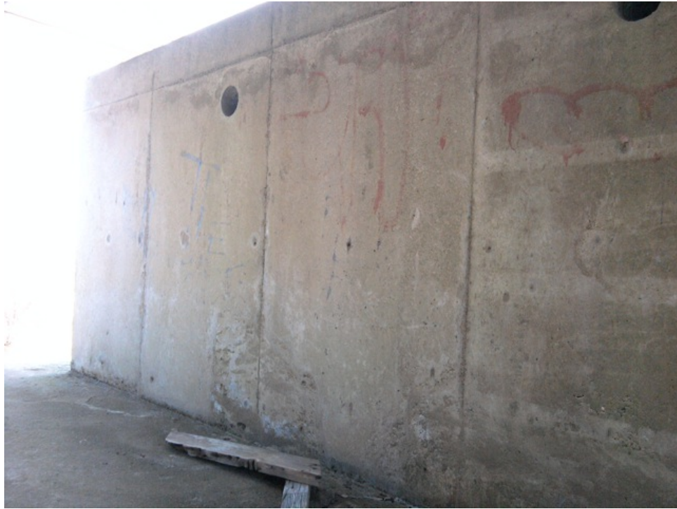
[Fig. 25] The south wall of Room 2-2, looking southeast. Note the false chimney remnant at the base of the wall.
