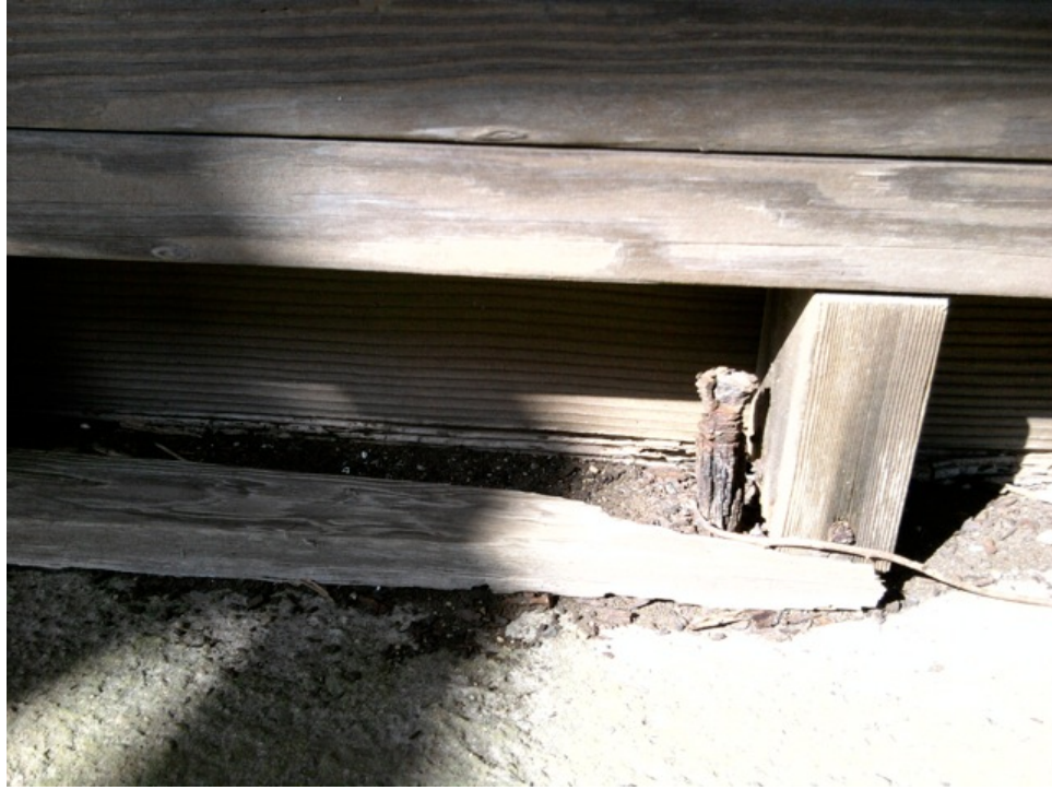
[Fig. 15] Detail of sill plate and roofing system, looking north. Note increased deterioration of wood and steel members.
