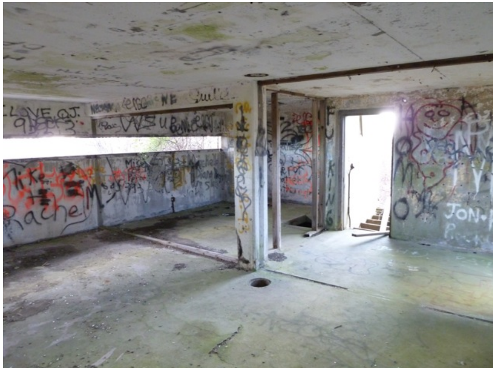
[Fig. 10] View of Room 1-1, looking southwest. Note the hole for a stove ductwork and original paint treatment under graffiti.
