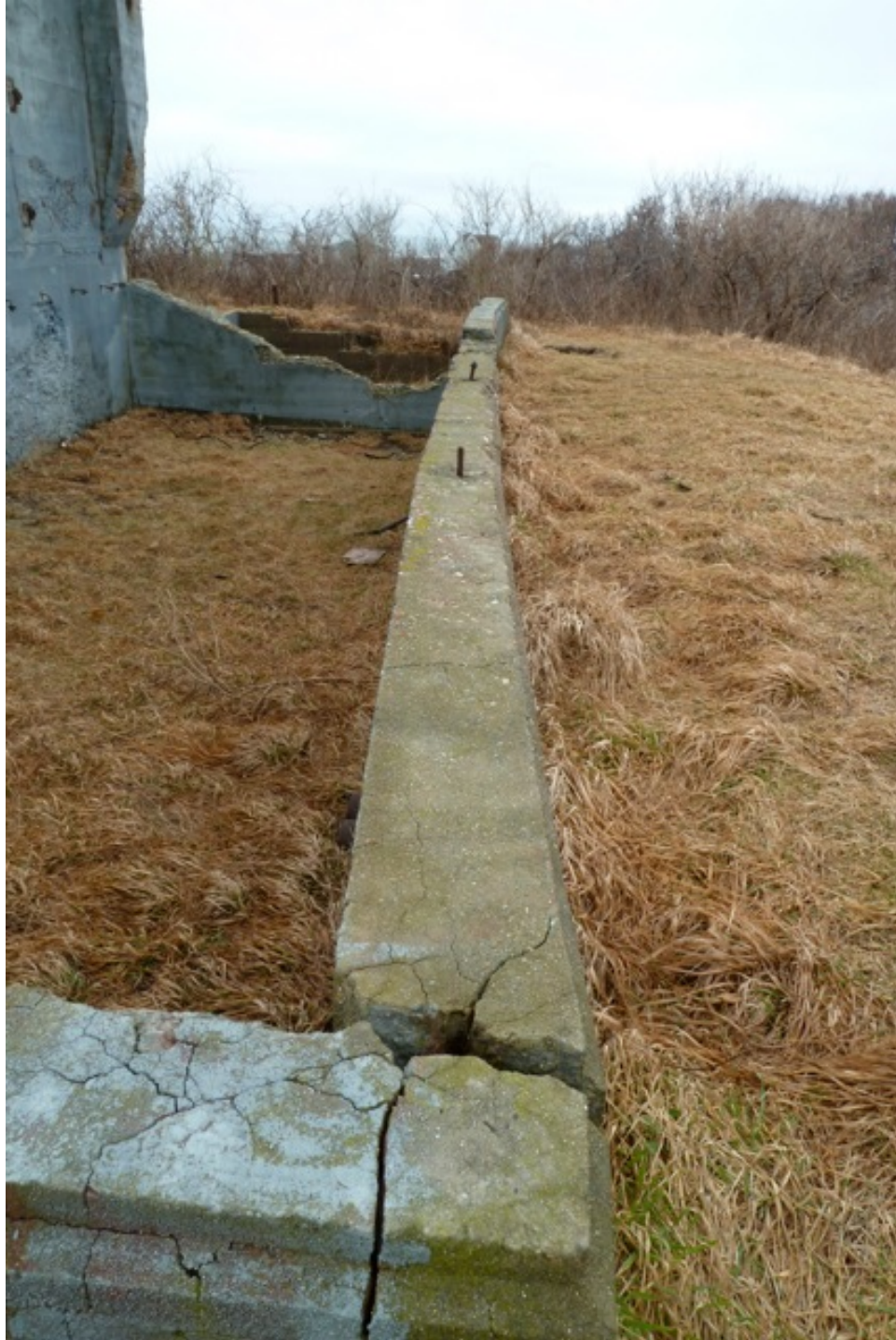
[Fig. 11] Detail of the northwest foundation wall, looking southwest. Note the bowing due to insufficiently retaining the change in ground level.
