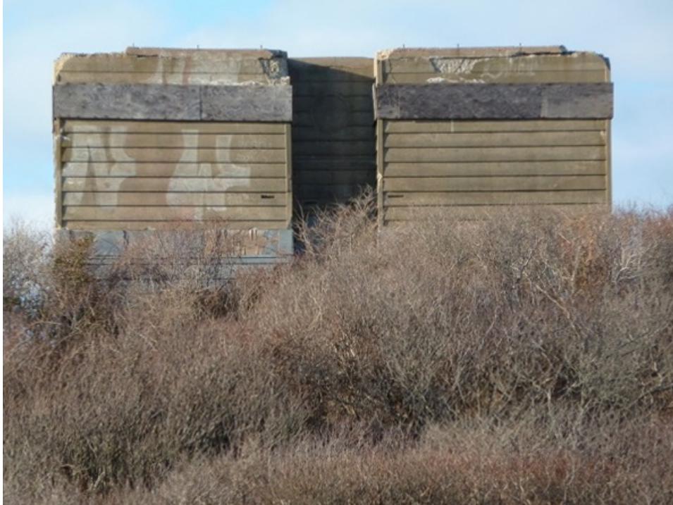
[Fig. 3] View of southeast elevation, looking northwest. Note the excessive erosion and cracking at the roofline.
