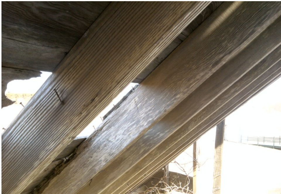
[Fig. 10] Detail of rafters, looking northeast. Note the occurrence of rot near holes in the roof.
