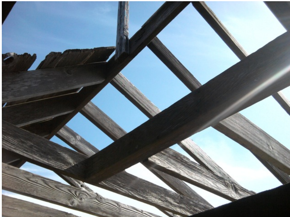
[Fig. 12] Detail of roof structure, facing southeast. Although weathered from exposure, the rafters have remained in good condition.
