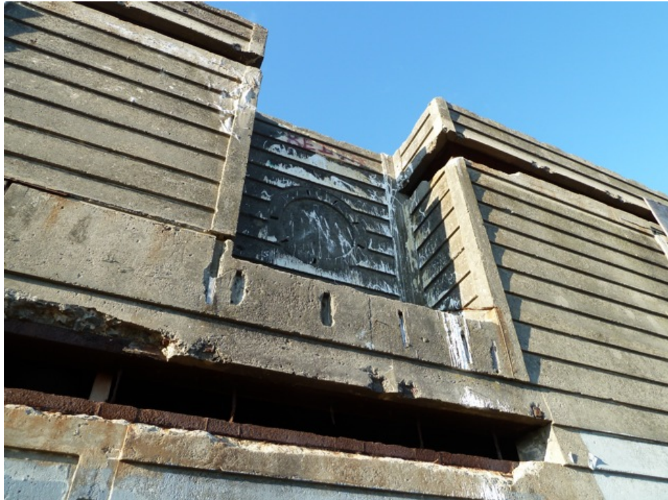
[Fig. 9] Detail of the south elevation, looking north. Note the paired concrete chipping above the ribbon windows, corroded steel within the ribbon windows, locations of wooden nailers, and formed concrete to mimic wooden clapboards.
