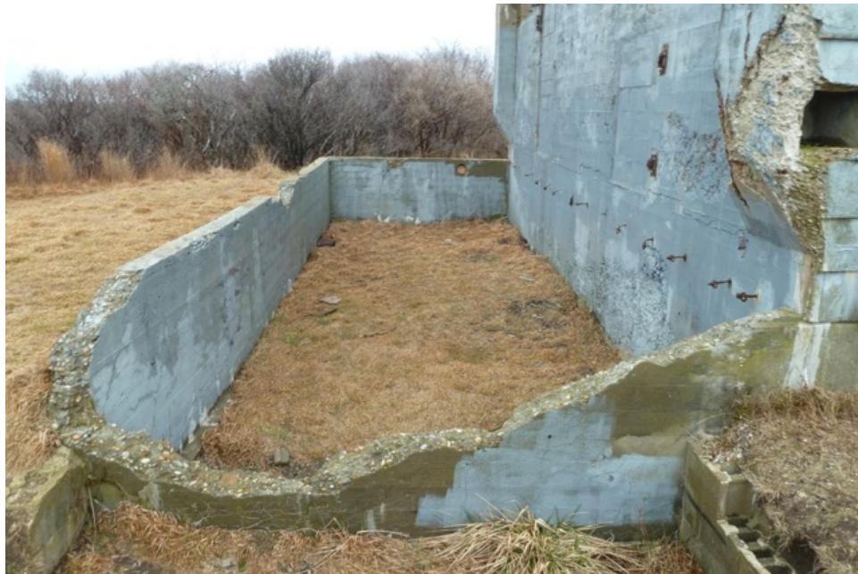
[Fig. 10] View of the southwest foundation wall, looking northeast. Note the excessive concrete erosion throughout.
