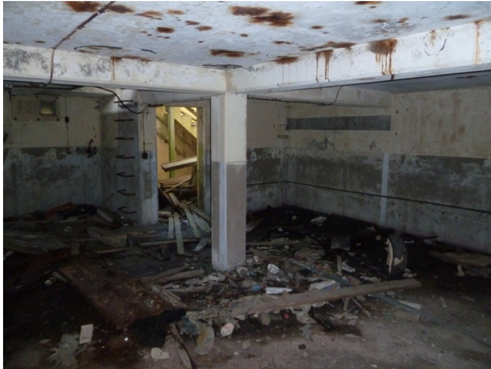
[Fig. 5] View of Room B-1, looking northwest. Note rust stains on the ceiling, debris, intact electrical conduits, ladder rungs, and original paint treatment.
