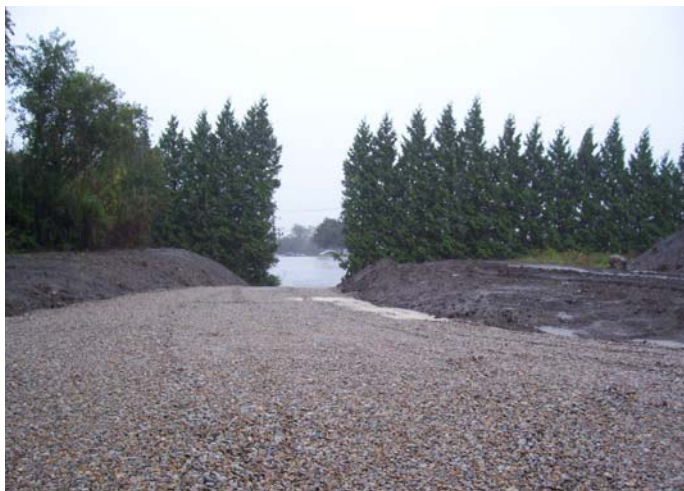
View of the Access Roadway from the Wind Turbine Site on the top of Fort Butts Hill in Portsmouth.
