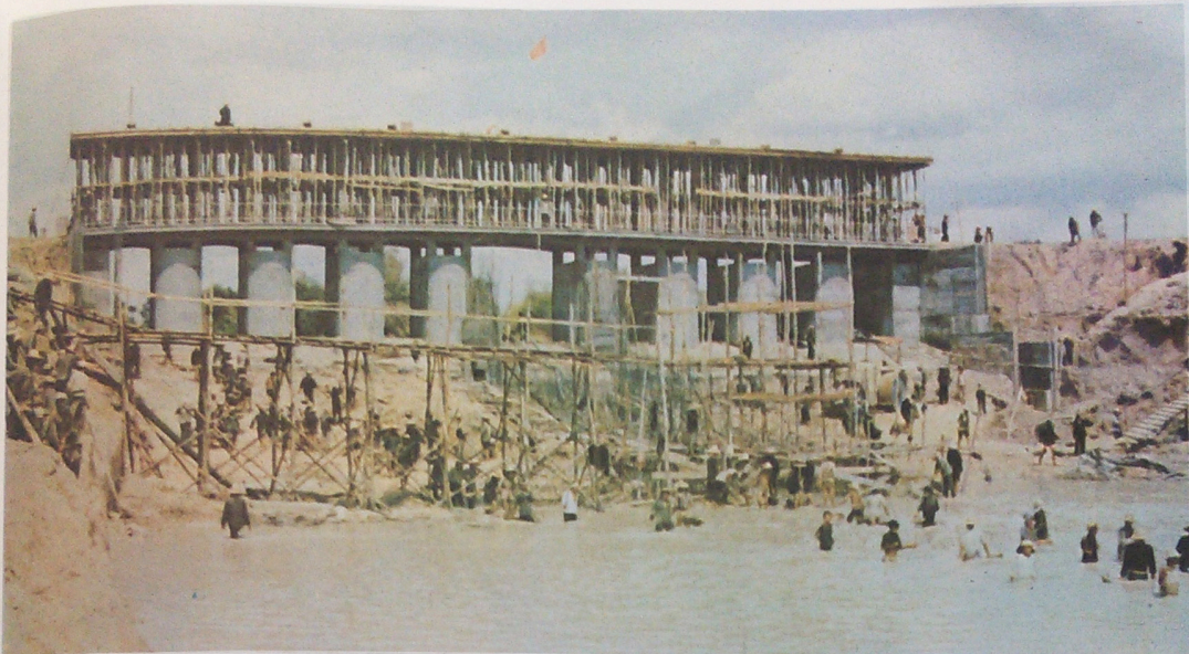
Dam on the Chinit river, province of Kompong Thom (Central region). The construction of this dam lasted five months from January to May 1977. The water of this dam can irrigate 20,000 hectares of rice-fields.
