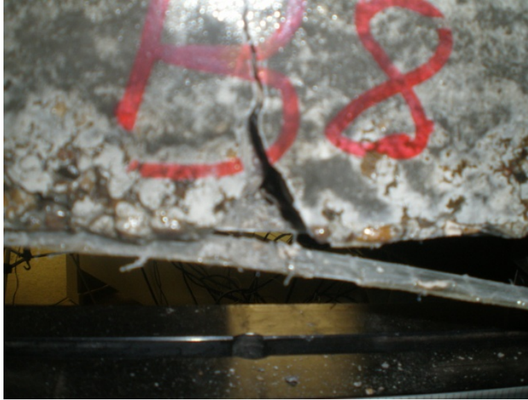
a) Concrete flexural crack and FRP delamination, B8
