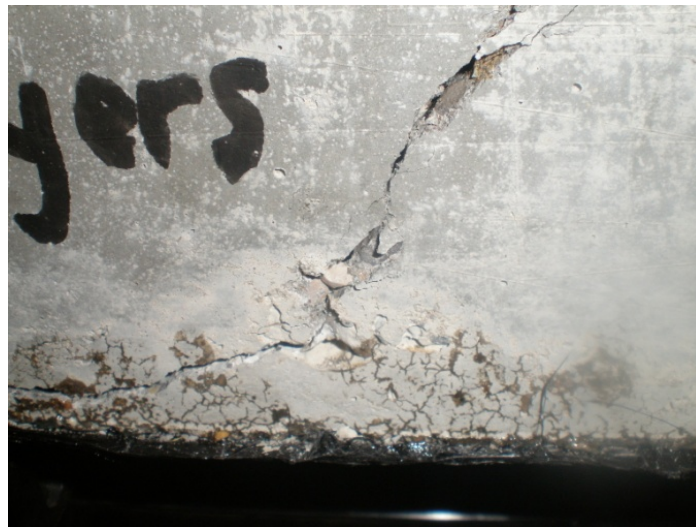
Figure 6.74: Shear failure of two layers Fyfe CFRP beam specimen, B3
