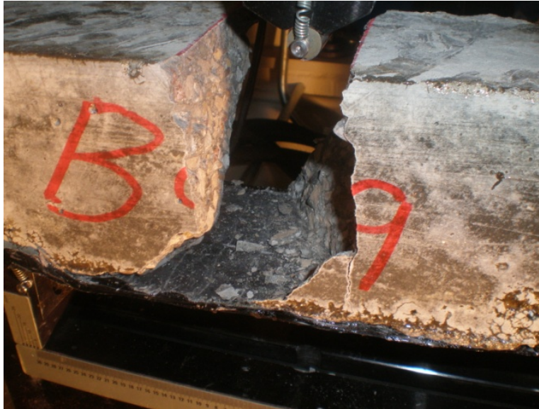
a) CFRP delamination, B9
