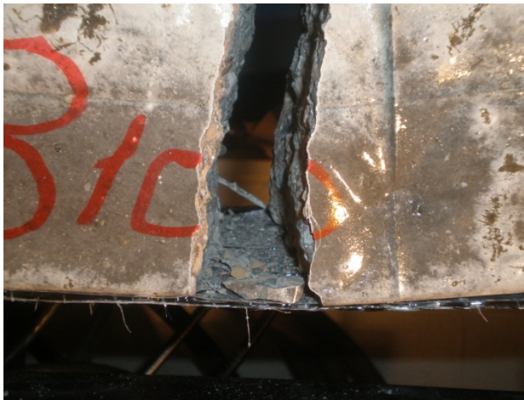
b) CFRP delamination, no rupture B10
