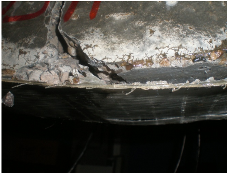
b) FRP Strips rip at the time of failure, B11
