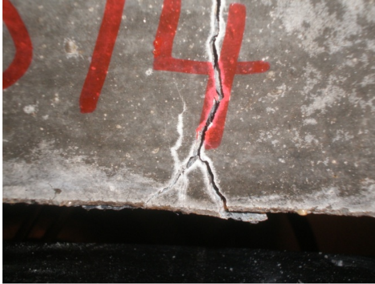
a) Concrete flexural crack, B14
