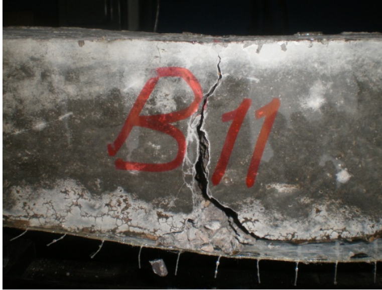
a) Concrete flexural crack and FRP delamination, B11
