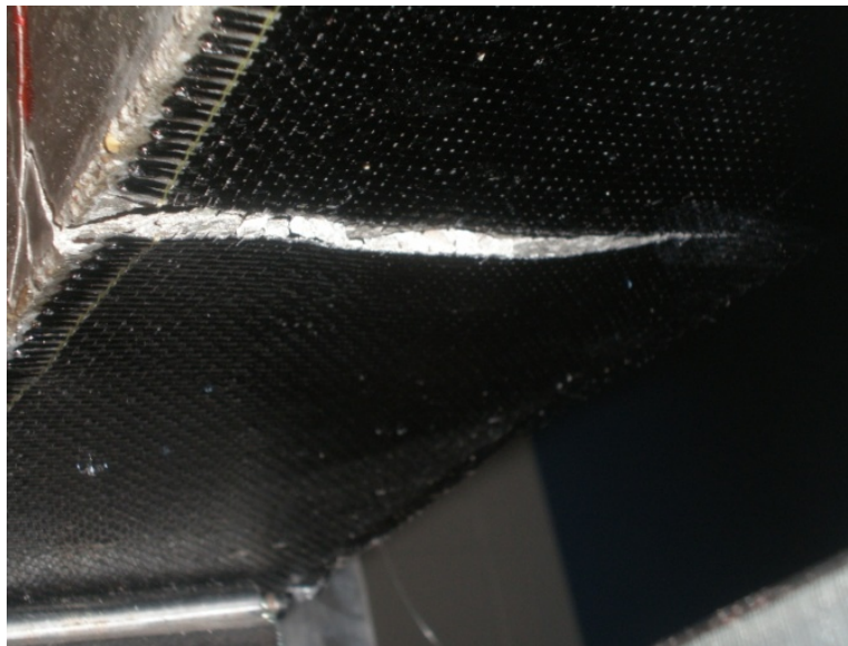
b) CFRP Rupture B14
