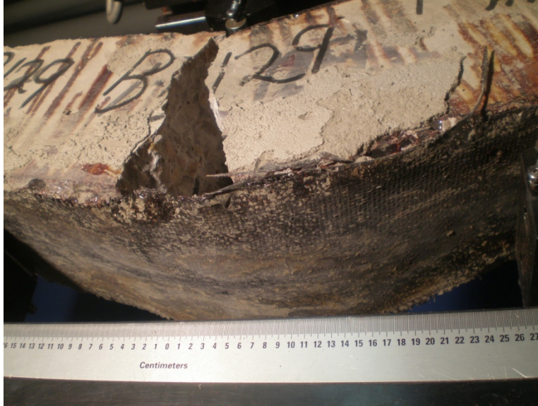
Figure 8.11: FRP delamination of B129, no rupture on the FRP surface
