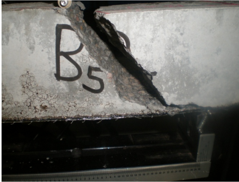
Figure 6.73: Shear failure with CFRP delamination, B5
