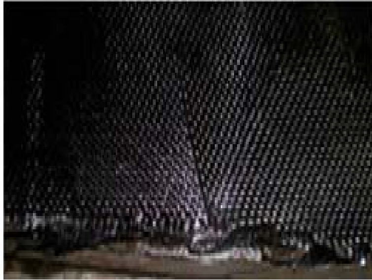
b) FRP rupture, beam B6
