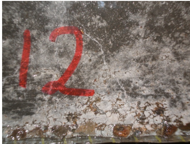
a) Concrete flexural crack followed by shear crack of specimen B12
