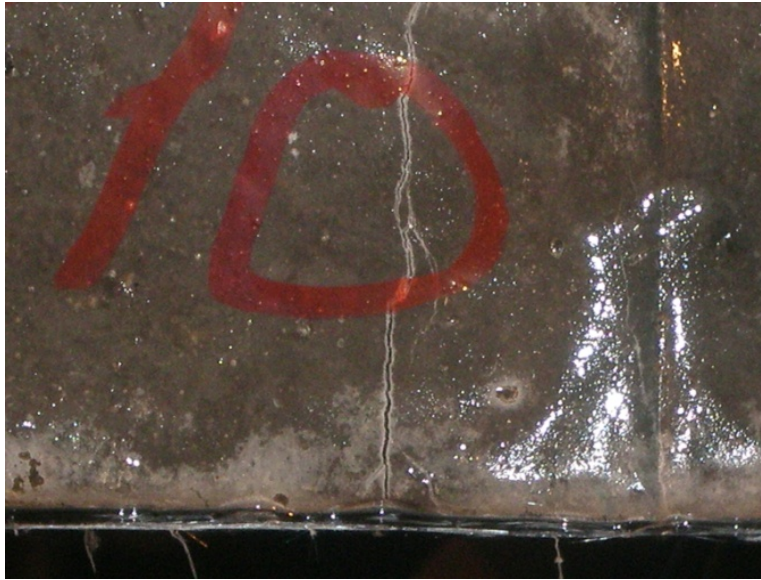
a) Concrete flexural crack, B10
