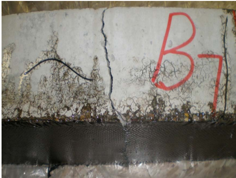
a) Concrete flexural crack, beam B7
