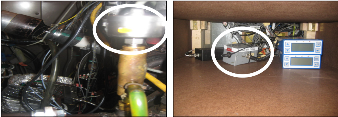
Figure 2.8 – Before turbocharger pressure transducer and its charge amplifier.
