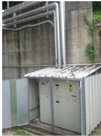
Figure 3. 11: heat pump installed near the Palacus sport palace
