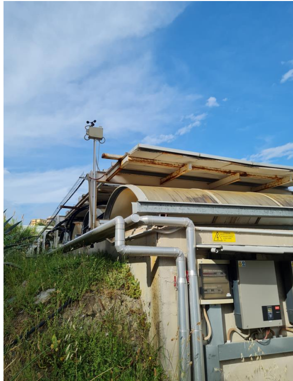
Figure 3. 22: weather station at the solar field – Palacus
