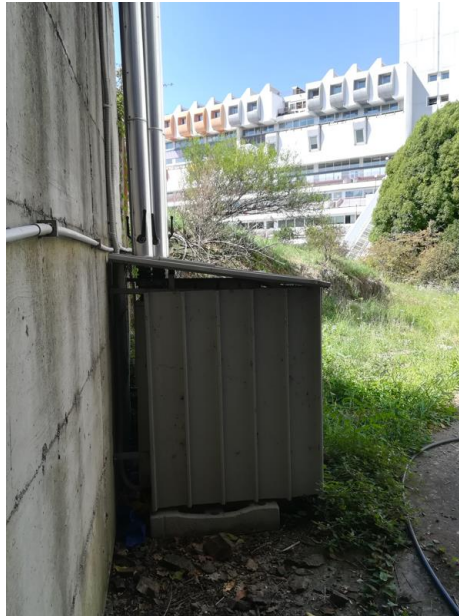
Figure 2. 5: solar assisted heat pump pilot plant with hybrid panels at Palacus – Genoa
