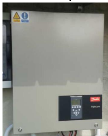
Figure 3. 9: one of the two 10 kW inverters installed near the solar field
