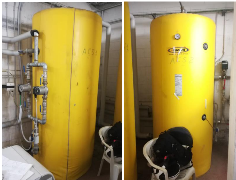
Figure 3. 17: domestic water storage tanks - DHW 1 on the left and DHW2 on the right
