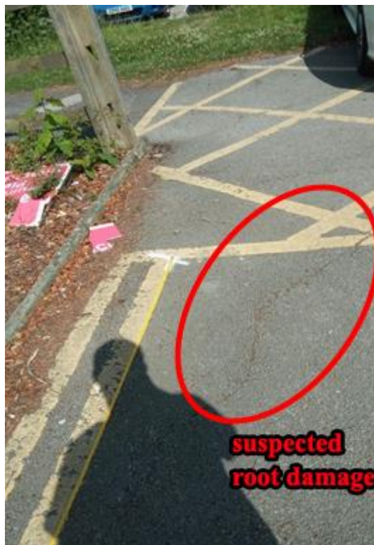
Figure 65. Image from the site with potential root damage visible on the surface.
