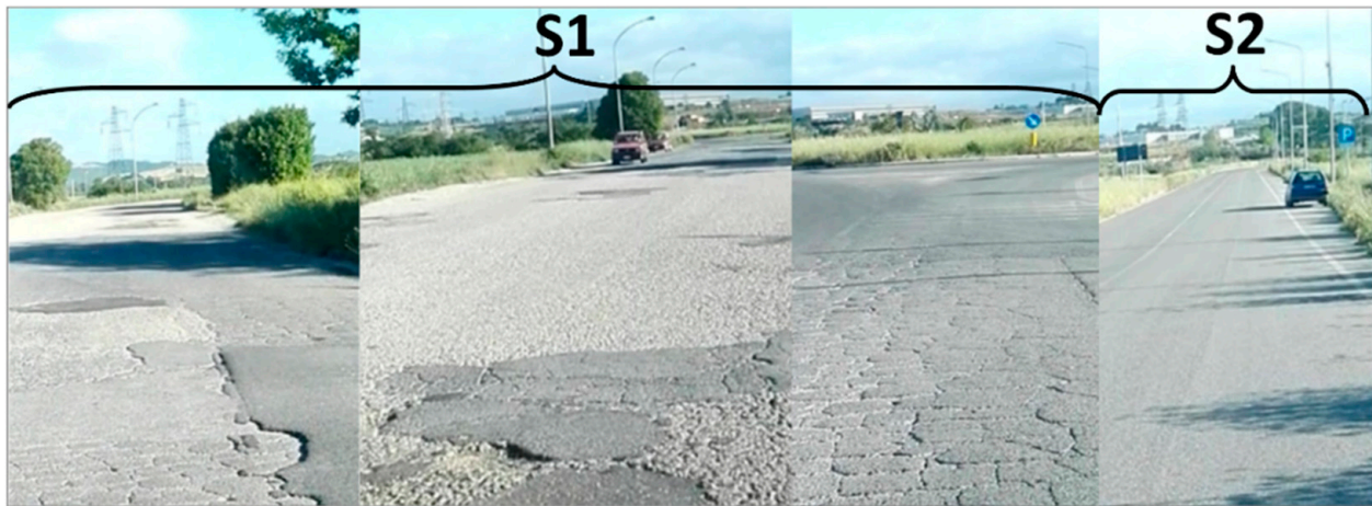
Figure 3. Alligator cracking, potholes, and patching all long Section 1 and non-distressed Section 2.
